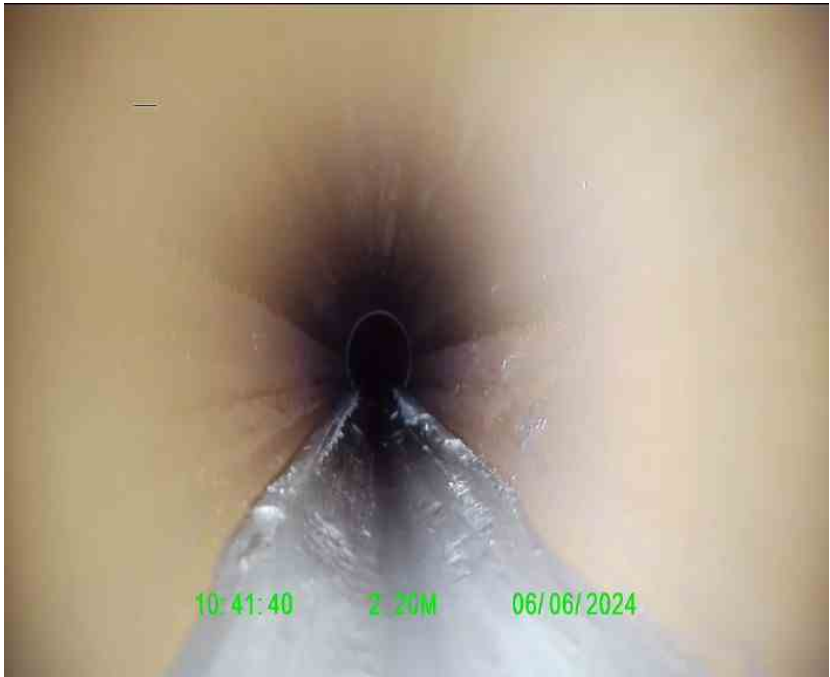
PIPE AX_7ac9f5c8-df0b-481d-99c8-0c3d1a5ac4ae_20240617_155228_607.jpg, 00:00:18, 2.20 m Settled deposits, hard or compacted, 15% cross-sectional area loss, start, Screed (Unable to remove with HPWJ)
