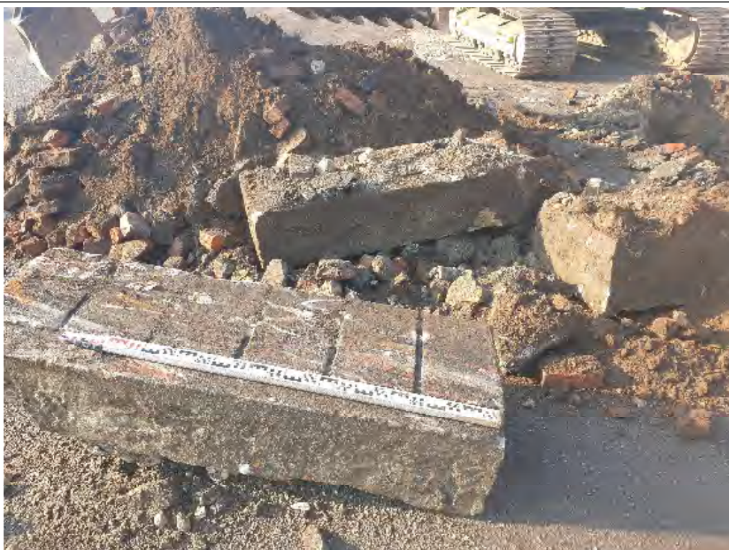
Photo No. 10: TPI04 Arisings
