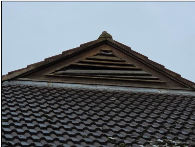
Photograph 12 showing deteriorated boards at southeastern elevation
