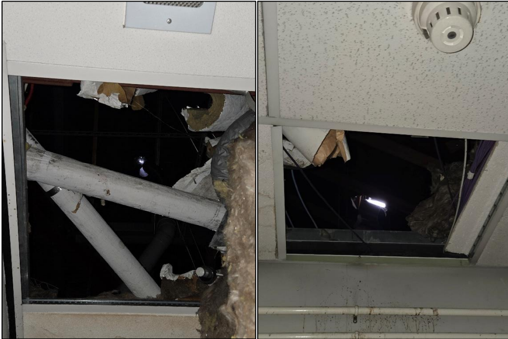
Photographs 14 &15 showing gaps in roof lining
