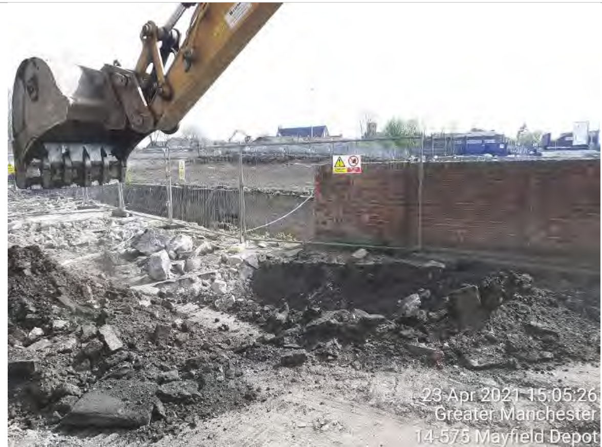
PLATE 5 PH314 HOTSPOT REMOVAL
