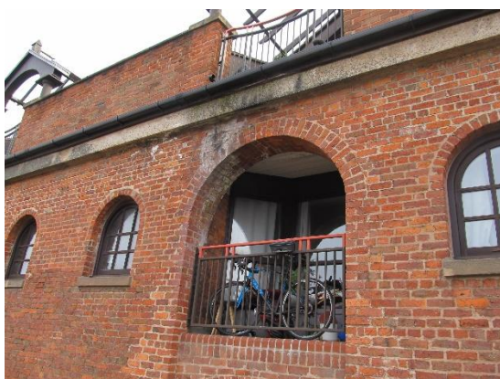
Evidence of prolonged surcharges from the eaves guttering affecting the brickwork below.
