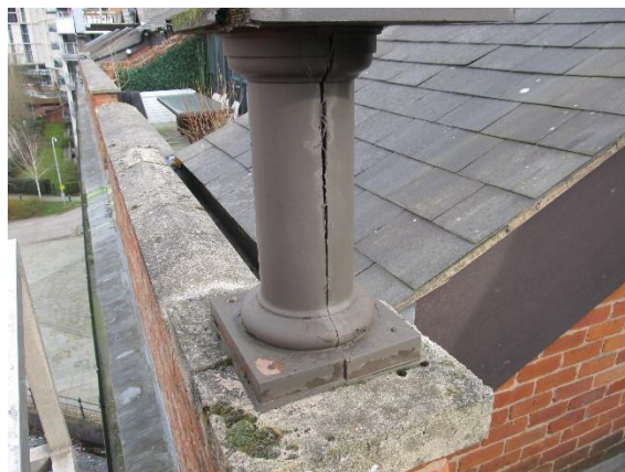
Open joints (typical) to GRP casings – potential source of rainwater to the parapet wall.
