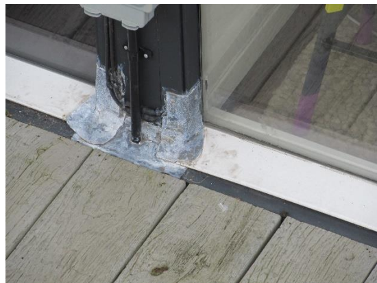
Retrospective lead saddle / bandage repair where electrical cables pass through the waterproofing to 504 Terrace.
