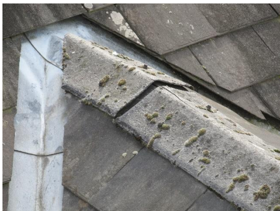
Split cement fibre ridge tiles and evidence elsewhere of slipped and missing slates to the rear roof slopes.
