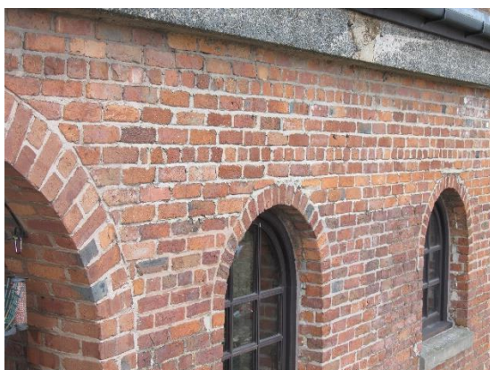
Solid masonry (English Garden Wall Bond) below concrete ring beam – note old rusted fixing bolt holes to former hopper head.
