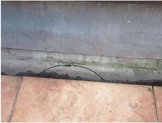
Typical example of cracked / fissured asphalt to the upstand skirting to 502 roof terrace.
