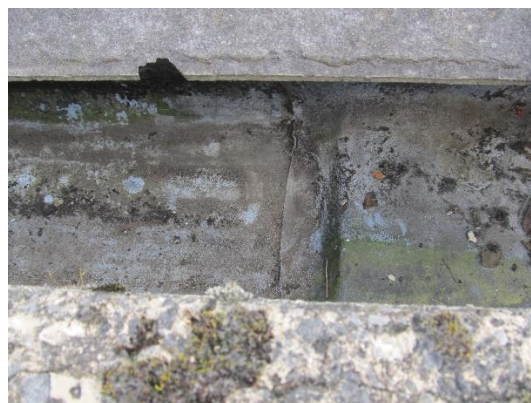
Potential for rainwater ingress to exploit the jointing to the lead sheet when the gutter is holding water.
