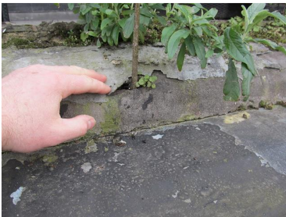
Obvious splits and defects to the asphalt to 505 terrace – remote from both 402 and 404 but included for context.
