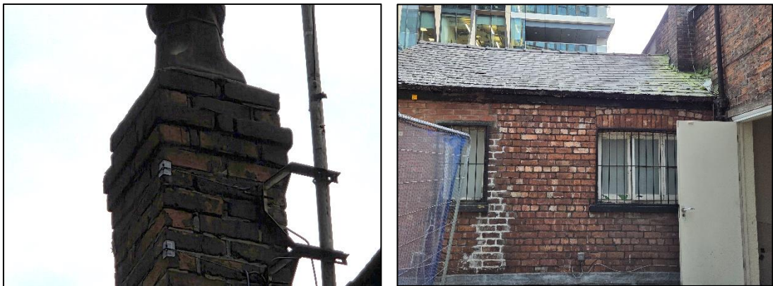
Plate 2. Lifted slate tiles and ridge tiles on the northern extension, and gaps in the chimney stack.
