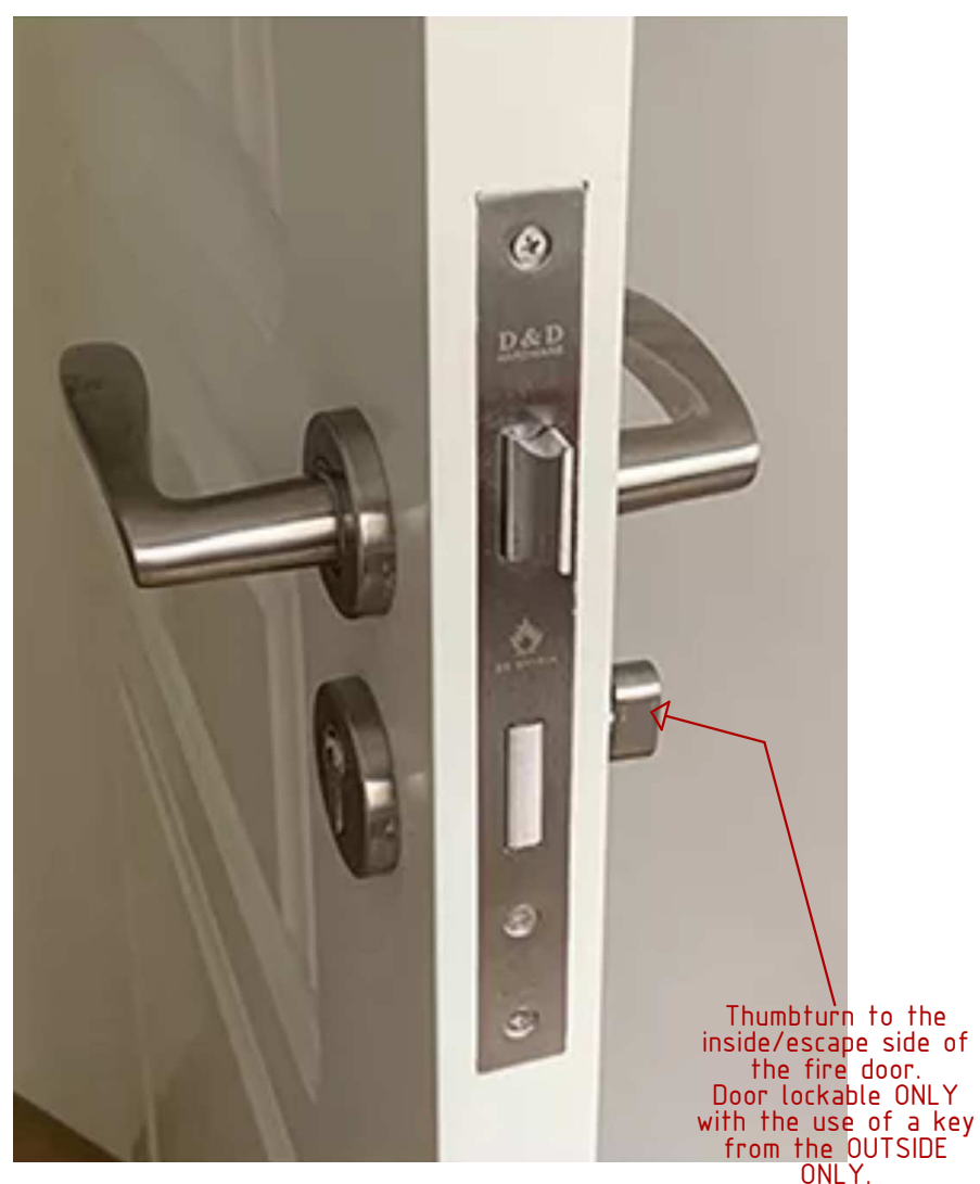
Typical Fire door Furniture.
