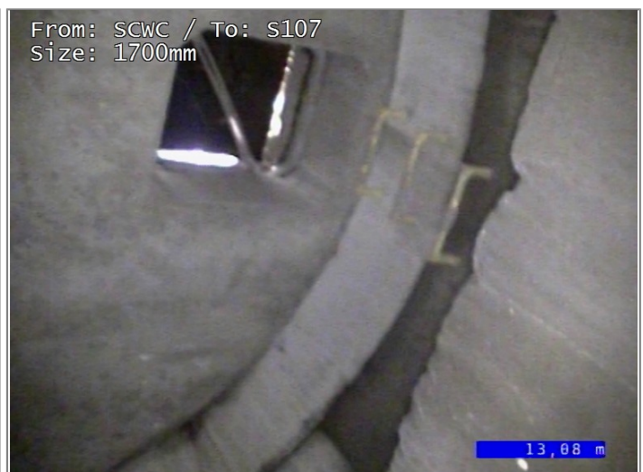
Finish node type, manhole, reference S107
