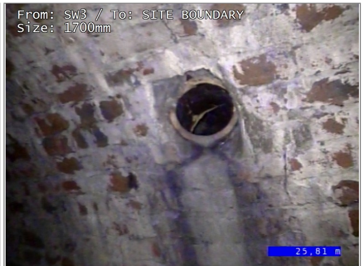
Connection other than junction, closed, at 2 o'clock, diameter 225mm
