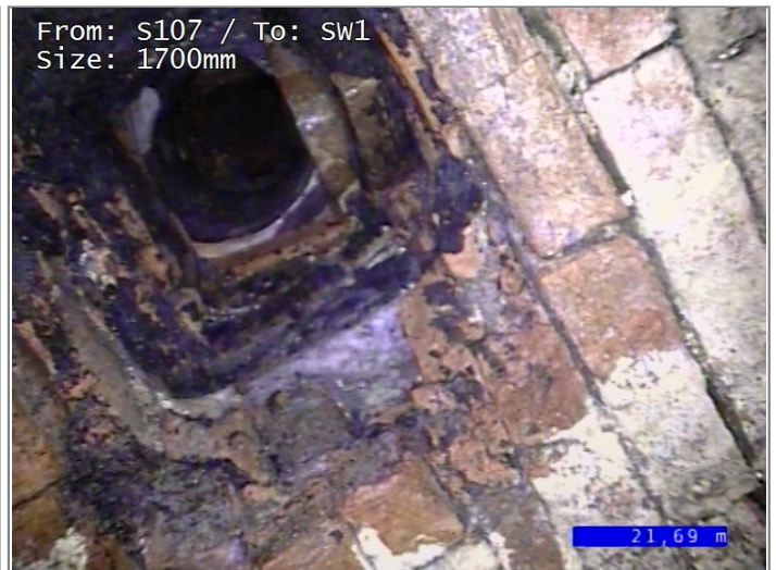
Junction at 12 o'clock, diameter 225mm
