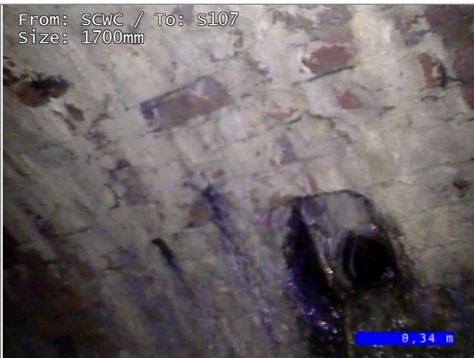
Junction at 4 o'clock, diameter 150mm
