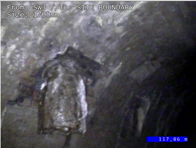
Connection intruding at 9 o'clock, diameter 225mm, intrusion 10%
