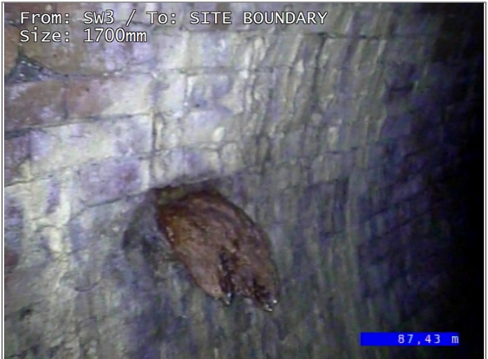
Junction at 8 o'clock, diameter 150mm
