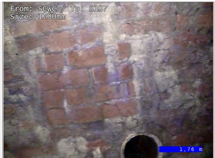
Connection other than junction at 8 o'clock, diameter 225mm
