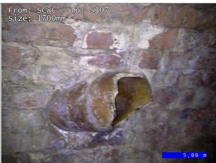
Connection intruding at 9 o'clock, diameter 150mm, intrusion 5%
