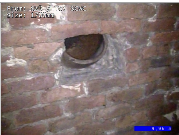
Connection other than junction, closed, at 10 o'clock, diameter 225mm
