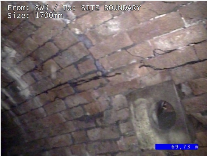
Junction at 4 o'clock, diameter 150mm
