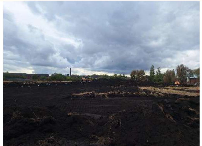
Photograph 8: Hazardous soils stockpile in sports pitch area
