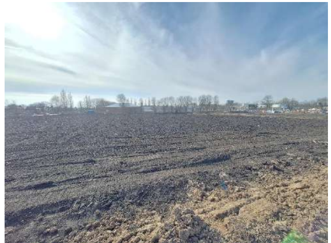
Photo 17: 20.03.25 – Hazardous topsoil placement
