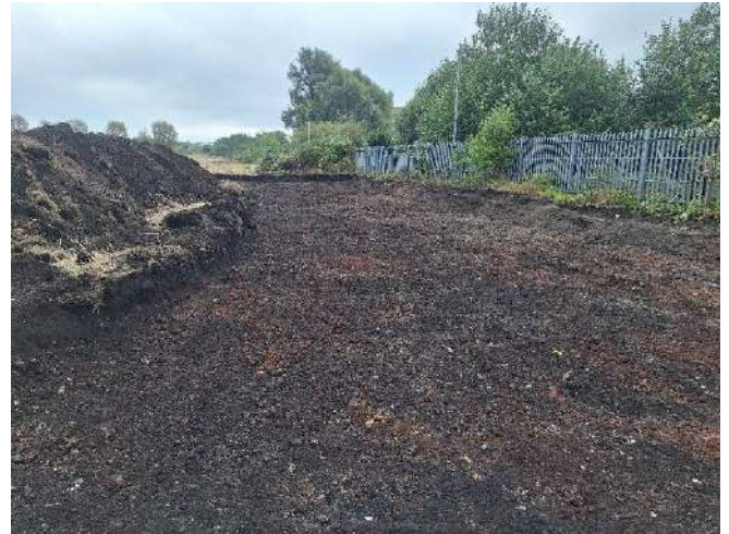
Photograph 4: Hazardous section following topsoil removal
