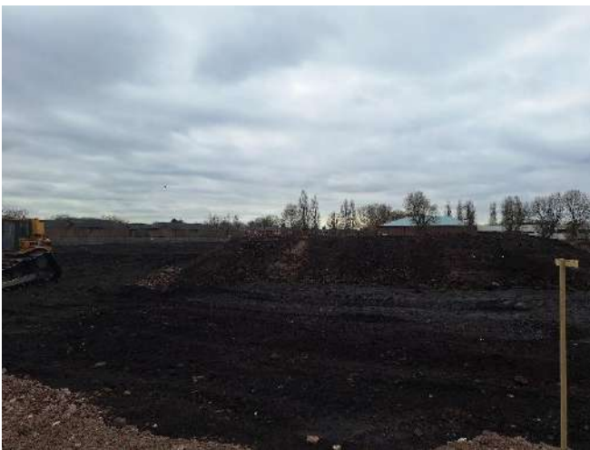
Photo 11: 03.03.25 – Hazardous topsoil placement
