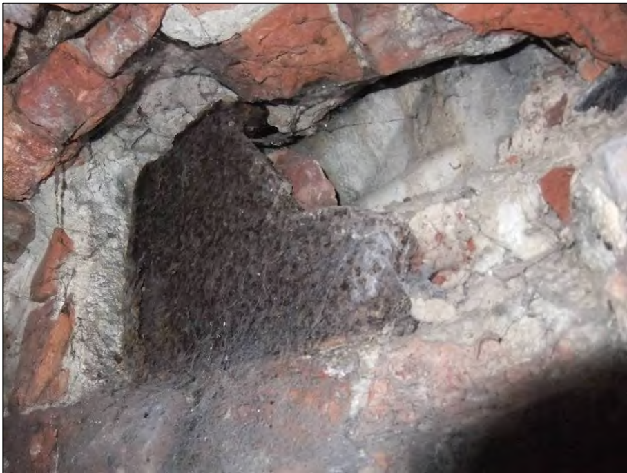
Plate 6 Culvert B24 example crevice at join between wall and roof with bat roost potential but no evidence
