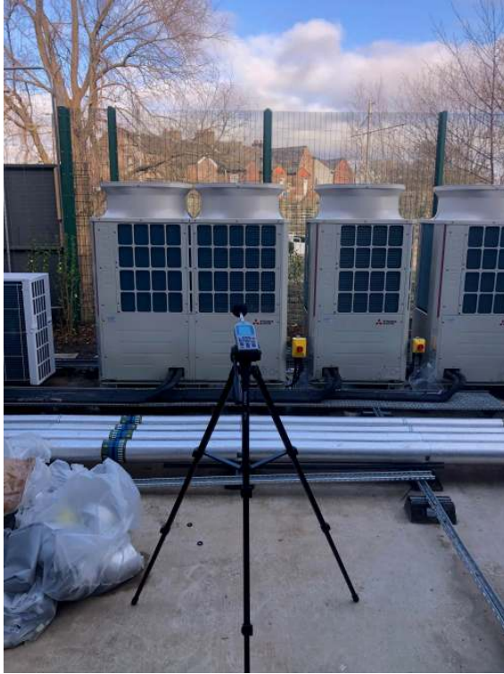
Figure 26: Location 4, 3 metres from the air handling units.
