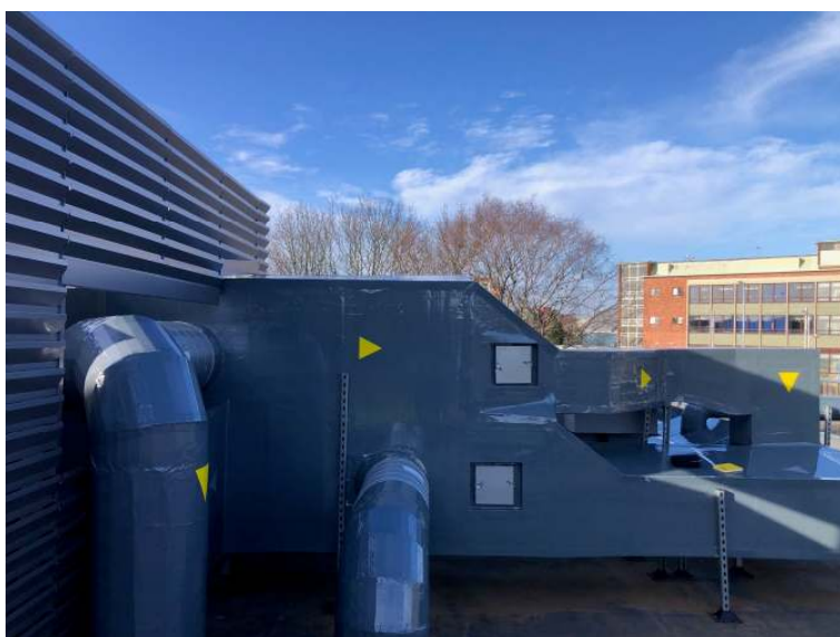
Figure 20: Lower roof plant.
