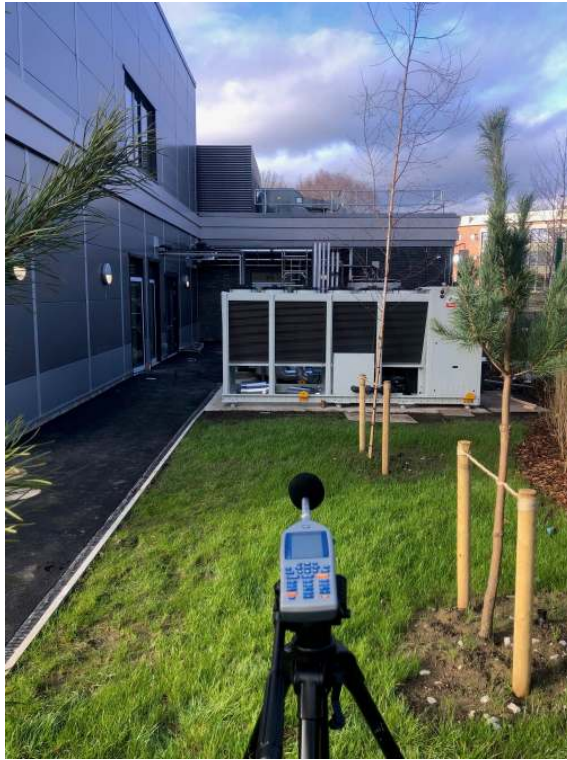
Figure 24: Location 3 10 metres from the air source heat pump.
