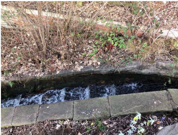
Figure 18: Free flowing water behind the lock.
