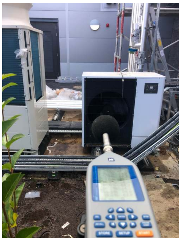
Figure 28: Location 5, 2 metres from the air handling units at the boundary fence.
