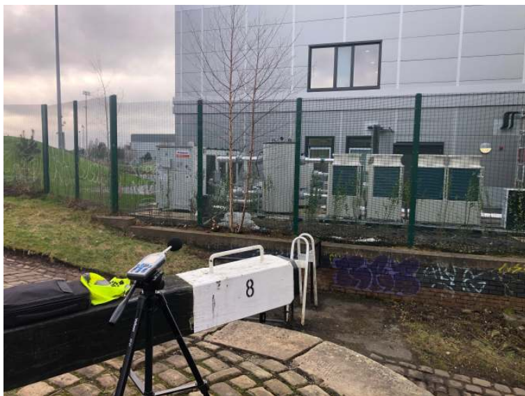
Figure 33: Measurement Location 6, 10 metres from the plant.
