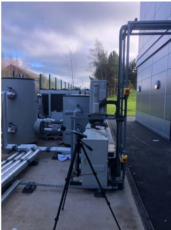
Figure 27: Location 4, 3 metres from the air handling units with the air source heat pump to the south.
