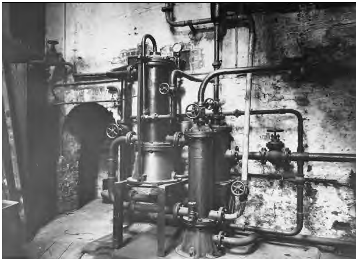
Plate 14: The Royle Calorifier at Mayfield Baths, 1902.
