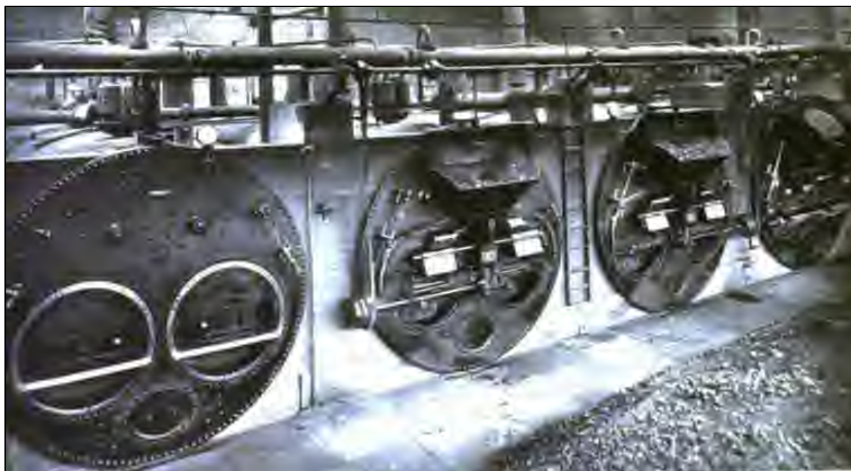
Plate 204: An example of a bank of Lancashire boilers, some fitted with automatic feeders (hoppers)
