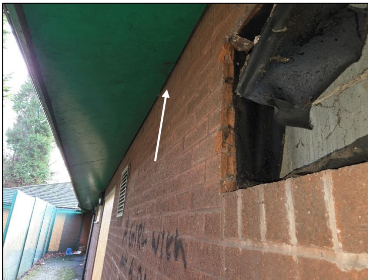
Photograph 3. Showing typical gap behind soffit.
