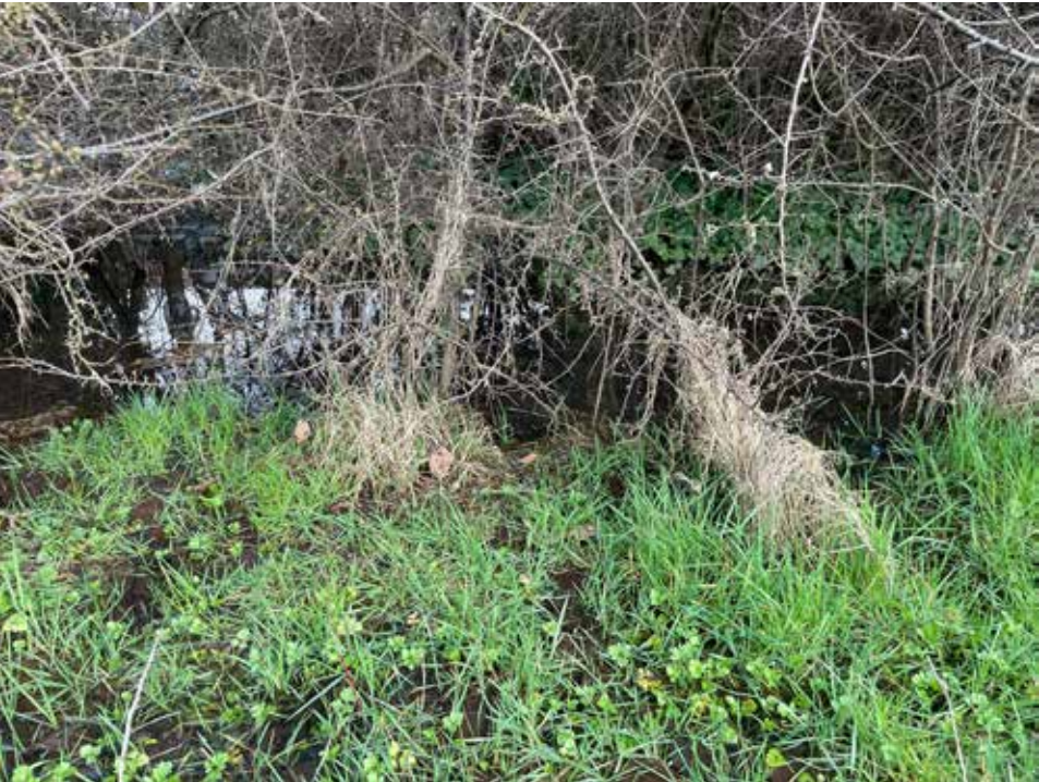
View of standing water underneath boundary blackthorn plantings
