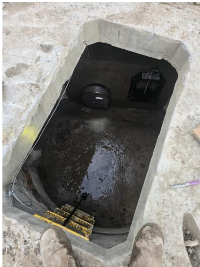
Photo 14: View of hydrobrake unit installed within manhole from cover slab.
