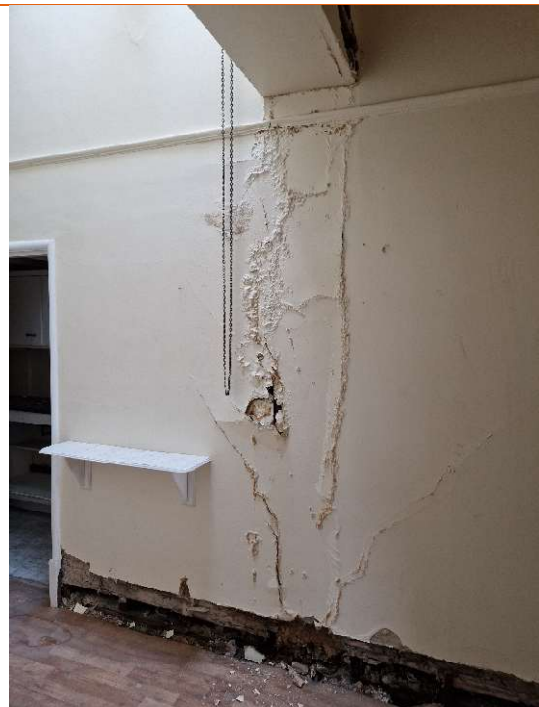
Photo 20 – Failed Internal Linings due to Water Ingress (First Floor)
