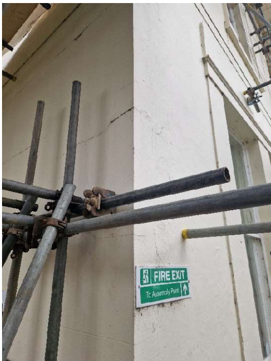
Photo 07 – Typical Cracking to External Render
