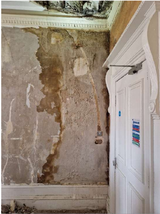
Photo 17 – Failed Plaster due to Water Ingress (First Floor)
