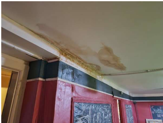
Photo 27 – Failed Ceiling Lining (Basement)
