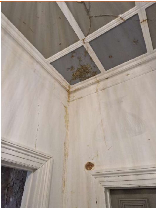
Photo 19 – Failed Internal Linings due to Water Ingress (First Floor)
