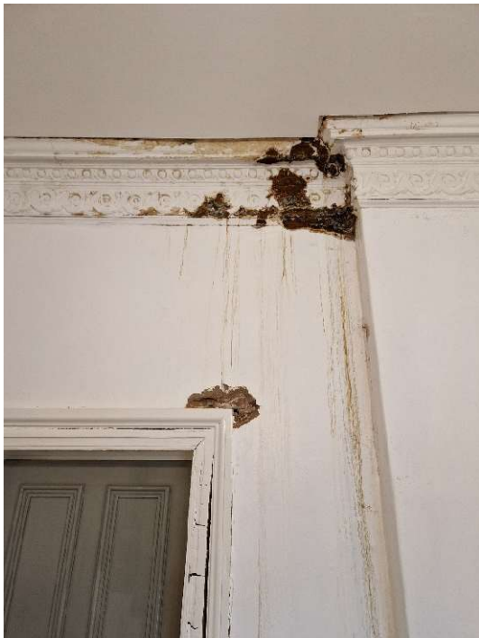
Photo 15 – Dry Rot Outbreak (Grond Floor)
