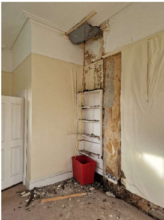
Photo 23 – Failed Internal Linings due to Water Ingress (First Floor)
