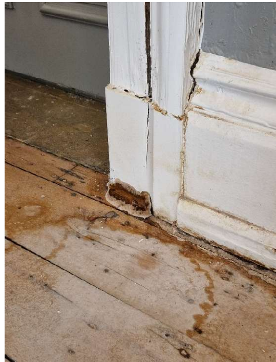
Photo 16 – Dry Rot Outbreak (Grond Floor)
