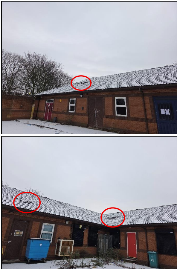
Photographs 6 & 7 showing areas of lifted roof tiles
