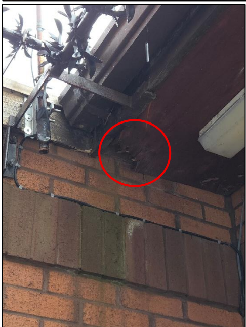
Photographs 8, 9, 10 & 11 showing gaps at end hip tiles and damaged and soffit board
