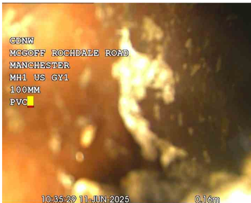
GY1X_7f4fee2f-65b9-41a1-b31a-f40cde79bea1_20250702_082329_146.jpg, 00:00:09, 0.16 m Settled deposits, coarse, 25% cross-sectional area loss
