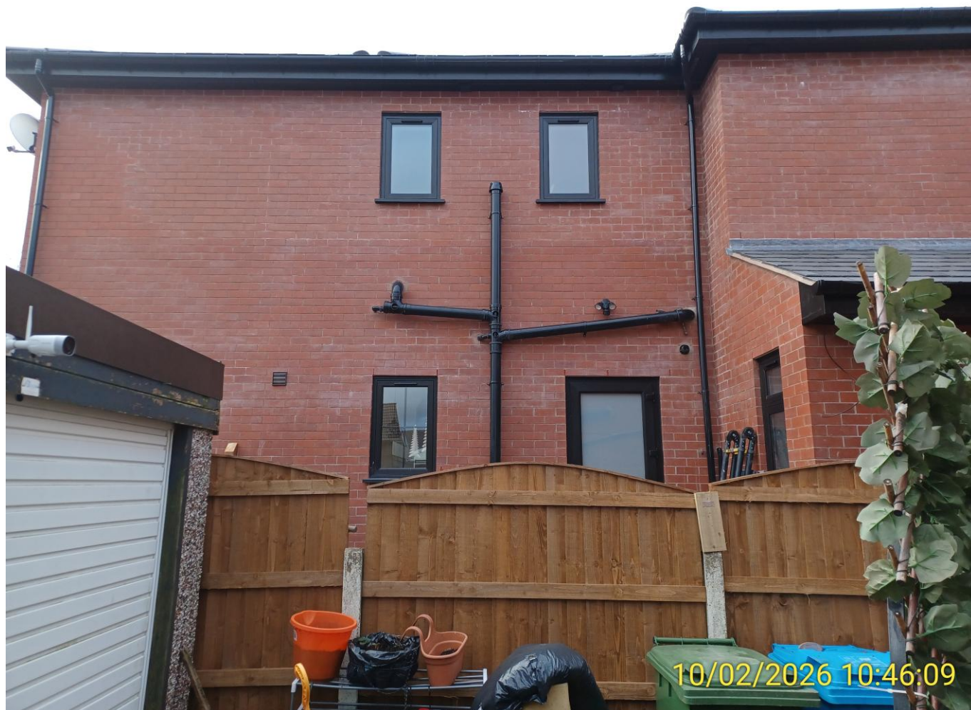
Photograph 2 Case officer site photograph of the ground and first floor windows as installed, taken on the date shown.
