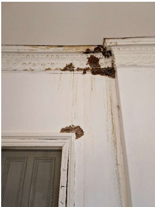
Photo 15 – Dry Rot Outbreak (Grond Floor)
