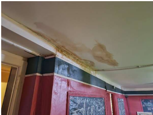
Photo 27 – Failed Ceiling Lining (Basement)
