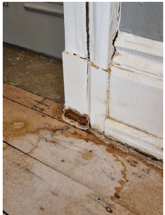
Photo 16 – Dry Rot Outbreak (Grond Floor)
