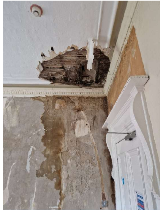
Photo 18 – Failed Plaster due to Water Ingress (First Floor)
