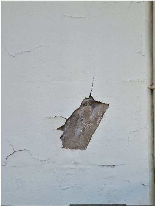
Photo 05 – Typical Section of Failed Render
