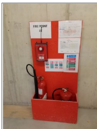
Fig 4: Example of typical onsite fire point
