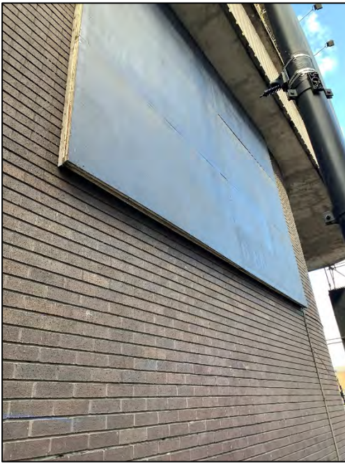
Photo 9 Wooden boarding on east face
