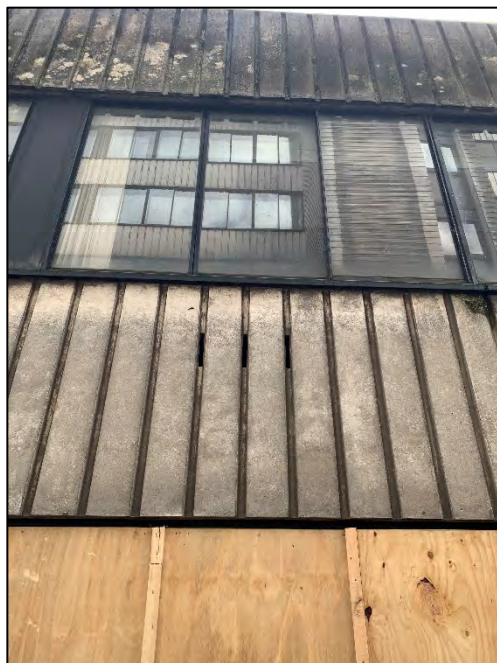
Photo 6 Gaps within concrete present on Premier House
