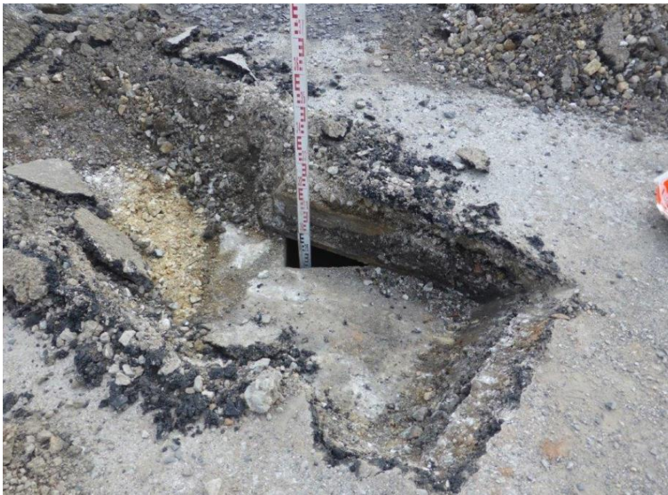
Figure 3-Abandoned chamber found during GI (1)
