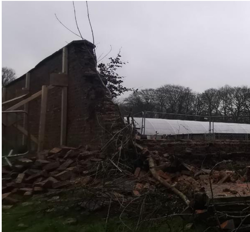
Photo 2 - Roots in collapsed wall
