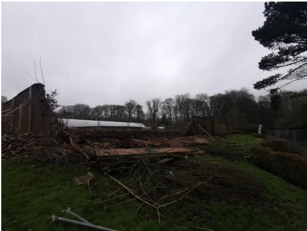
Photo 1 - Garden Centre Collapsed Wall
