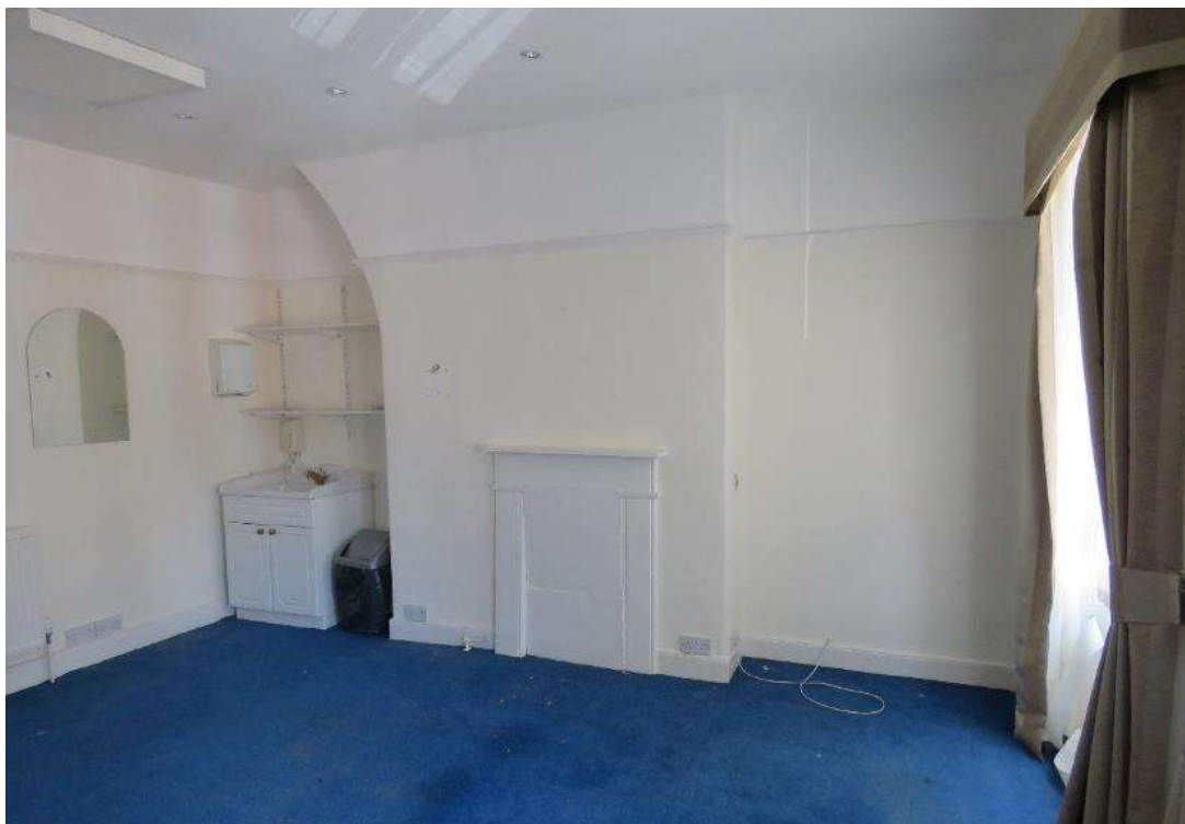
Figure 35 – A former servant's bedroom (Room 12), denoted by the use of simple skirtings, picture rail and fire surround (a surviving cast iron hob grate, though damaged, has been found concealed behind modern boarding).
