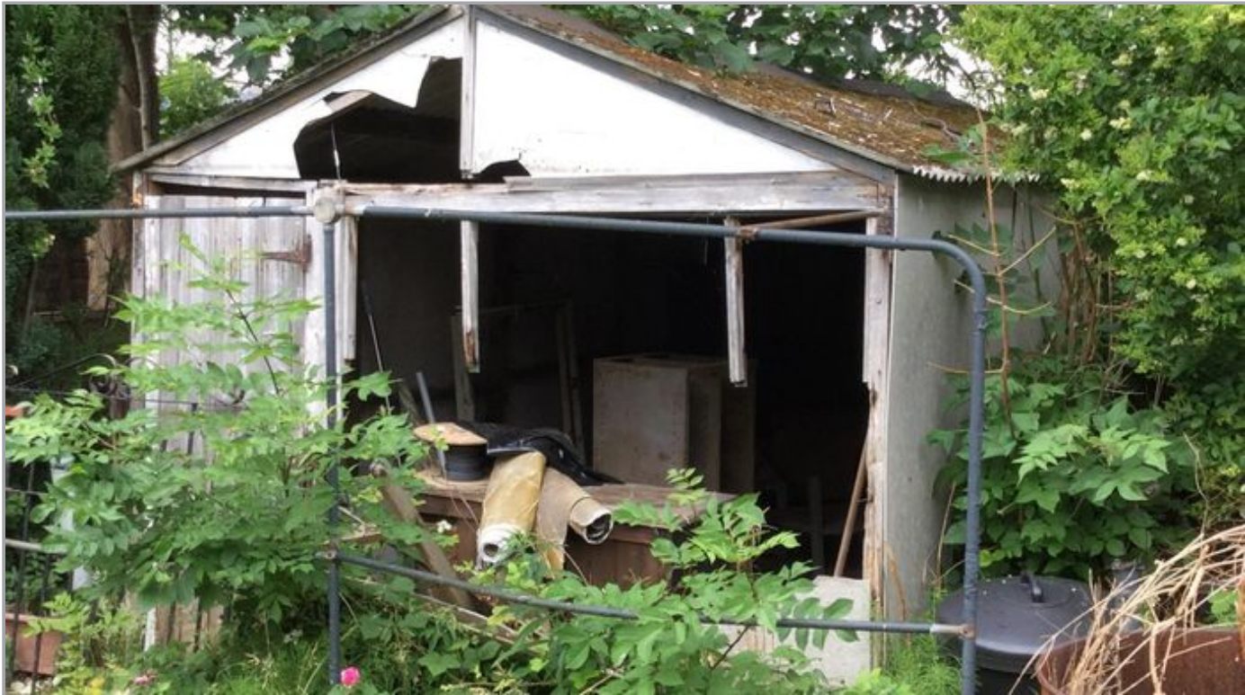
External store likely to be constructed of Asbestos panelling
