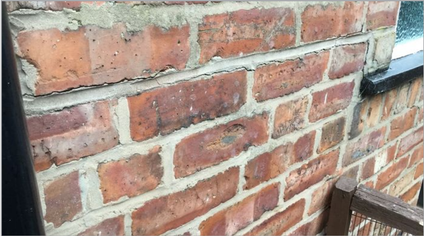
Horizontal cracking to wall of utility area
