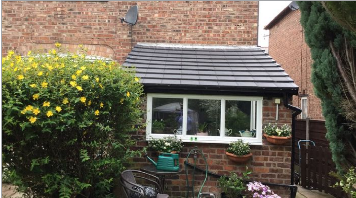
Slight sagging of utility room roof structure
