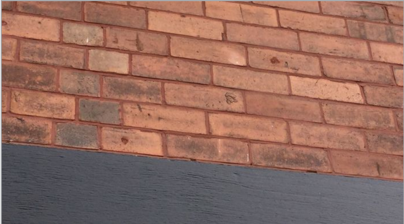
Plugged holes indicative of cavity wall ties
