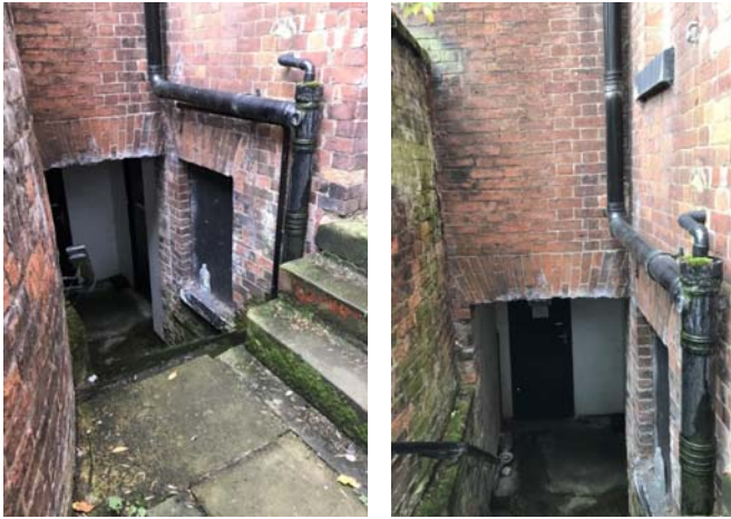
Leaking downpipes and stacks
