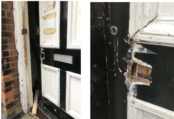
Damage to timber panelled doors and frames
