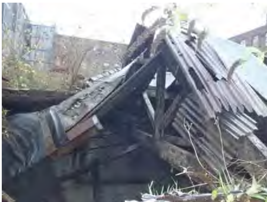
Photograph 14 – Derelict building roof in north of Site; suspected ACM panels
