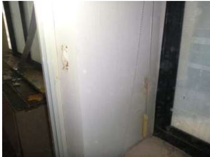
Concrete and Plaster to Column C4
