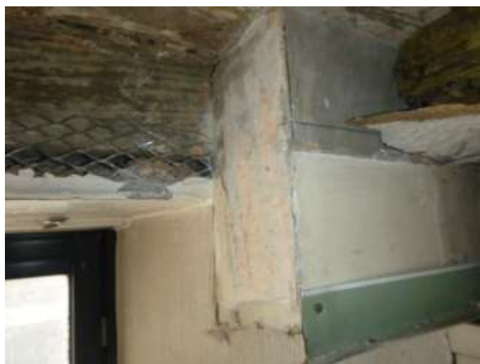
Concrete and Plaster to Beam at Top of Column C1
