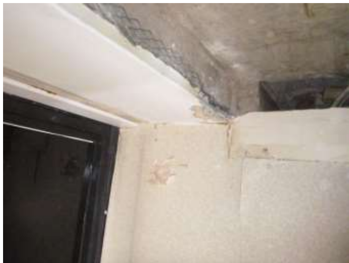
Concrete and Plaster to Beam at Top of Column C2
