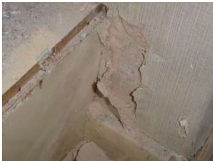
Concrete and Plaster to Column C7
