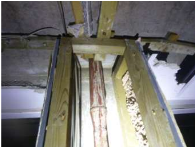
Non-Insulated Pipe in Boxing to Column C2
