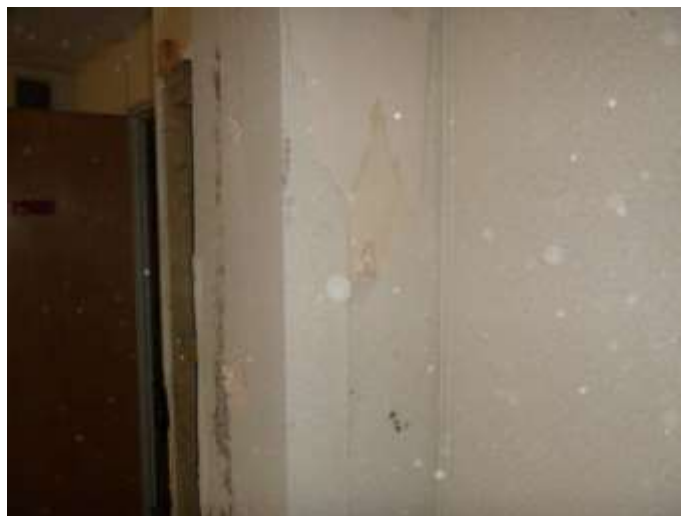
Concrete and Plaster to Column C8
