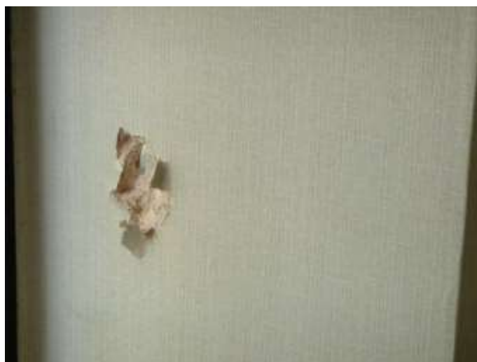
Concrete and Plaster to Column C7
