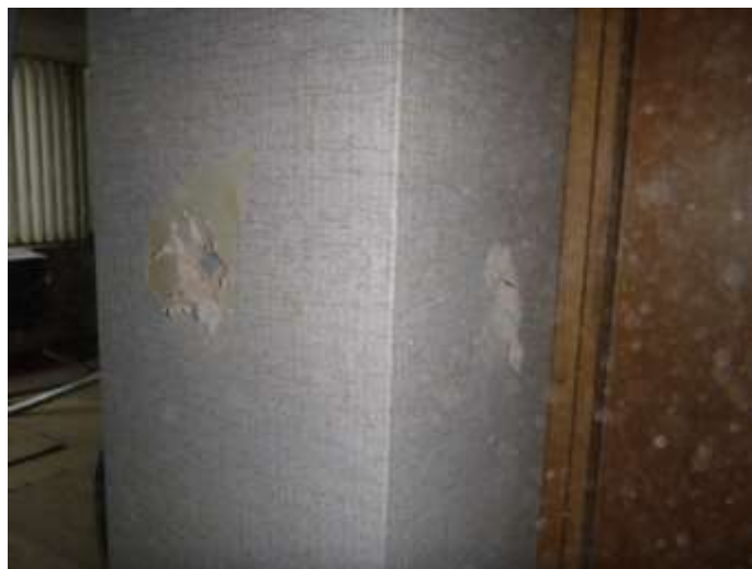
Concrete and Plaster to Column C5
