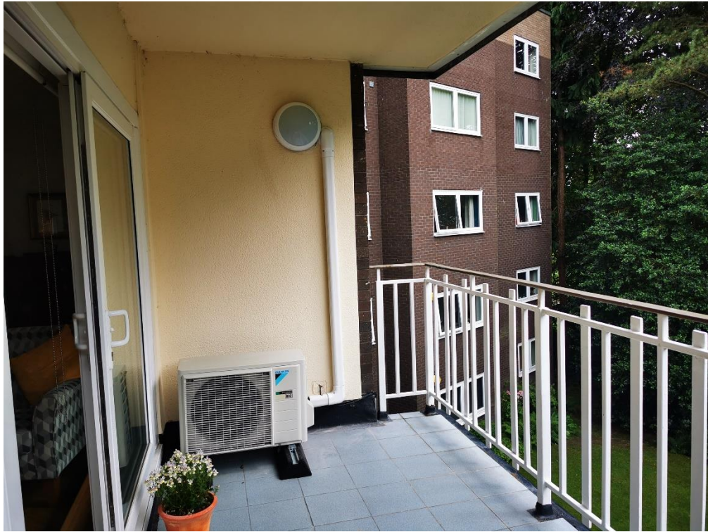
Photo showing the installed 1No. condenser unit
