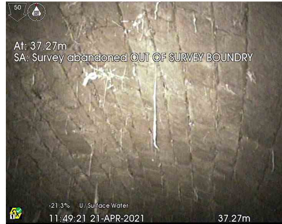
2_37-27m_114921.jpg, 00:09:34, 37.27 m Survey abandoned, OUT OF SURVEY BOUNDRY
