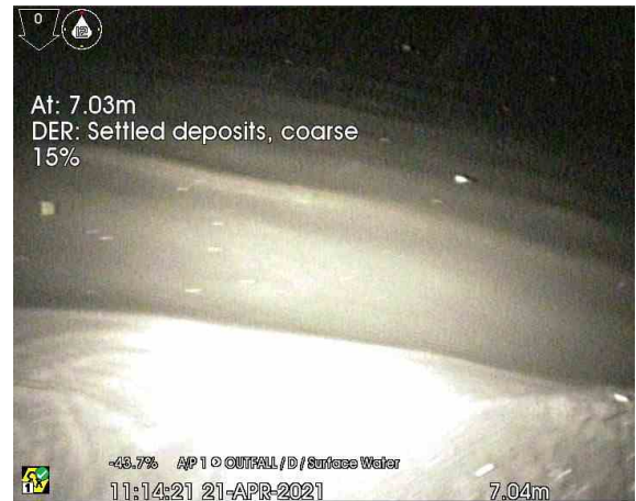
1_7-04m_111421.jpg, 00:00:52, 7.04 m Settled deposits, coarse, 15% cross-sectional area loss
