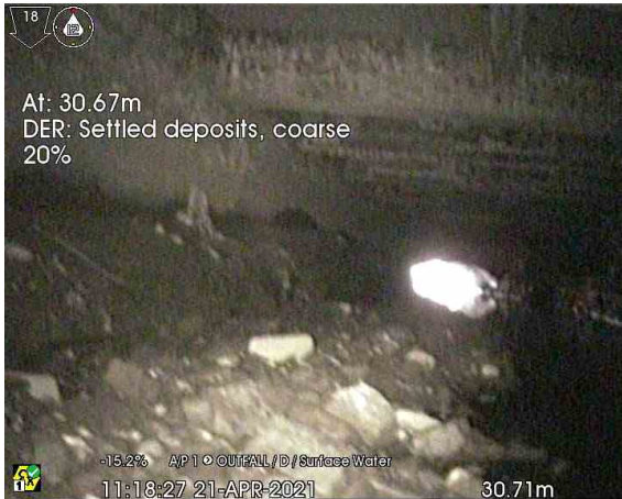
1_30-78m_111827.jpg, 00:03:47, 30.78 m Settled deposits, coarse, 20% cross-sectional area loss
