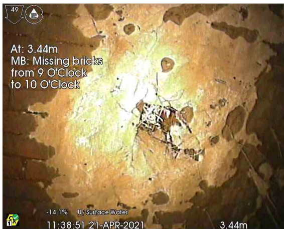
2_3-44m_113851.jpg, 00:00:53, 3.44 m Missing bricks from 9 o'clock to 10 o'clock
