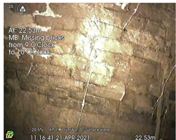
1_22-53m_111641.jpg, 00:02:49, 22.53 m Missing bricks from 9 o'clock to 10 o'clock
