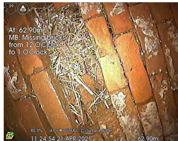
1_62-90m_112454.jpg, 00:08:20, 62.90 m Missing bricks from 12 o'clock to 1 o'clock
