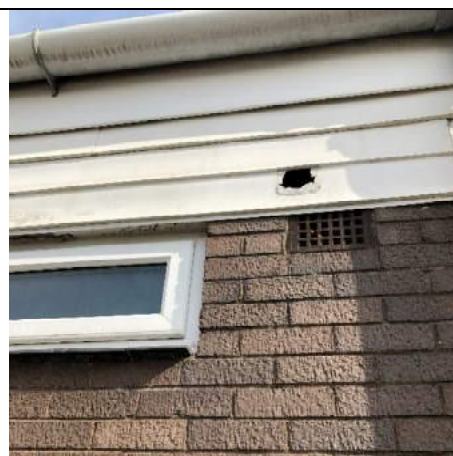
Photo 10: Hole present in weatherboard. Does not lead anywhere.
