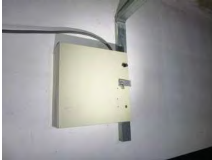
Modern Electrical Equipment to Upper Level
