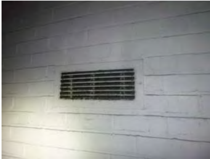
Metal Duct Grates to Walls
