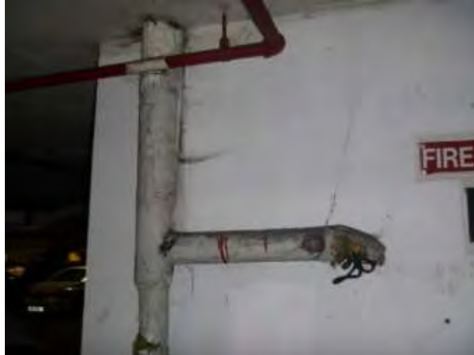
Rockwool Pipe Insulation near Electrical Switchgear – Mid Level
