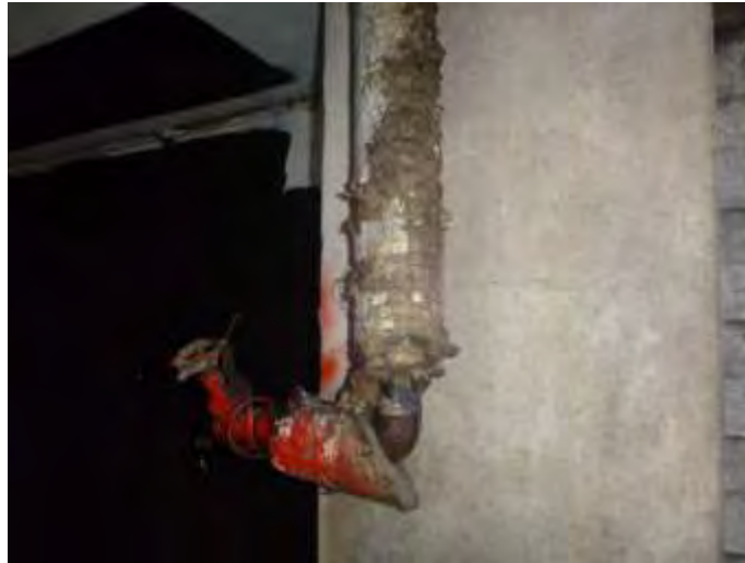
Rockwool Insulation to Pipes adjacent to Exterior Wall
