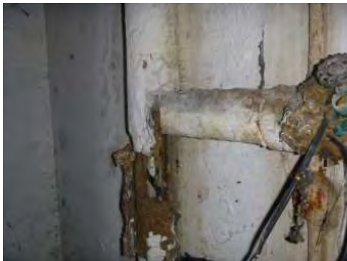
Rockwool Pipe Insulation near Roller Shutter Door – Mid Level
