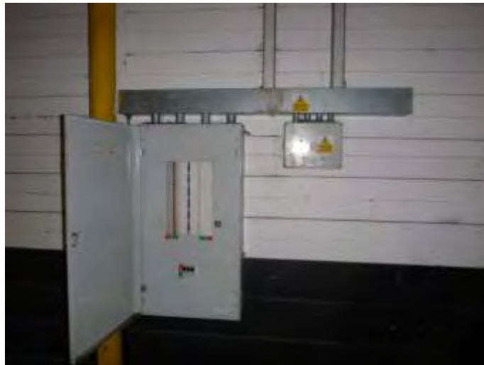
Modern Electrical Switchgear
