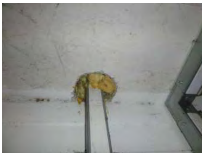
Foam to Pipe Egress Points
