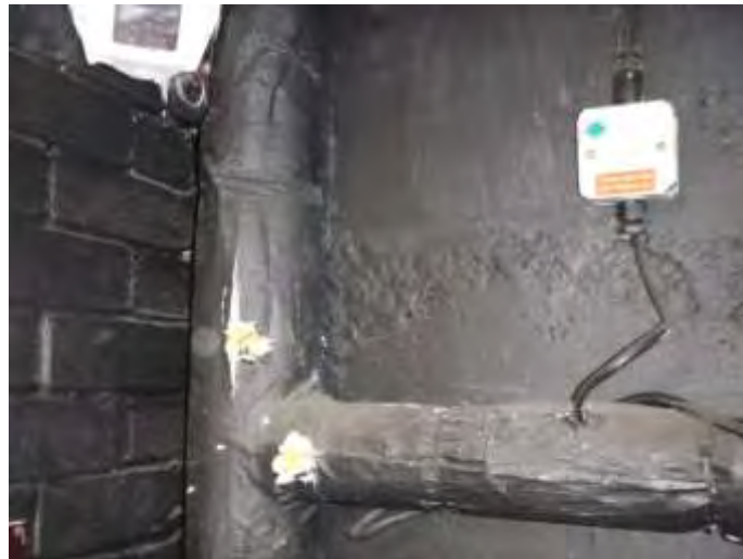
Rockwool Pipe Insulation adjacent to Hotel Lift
