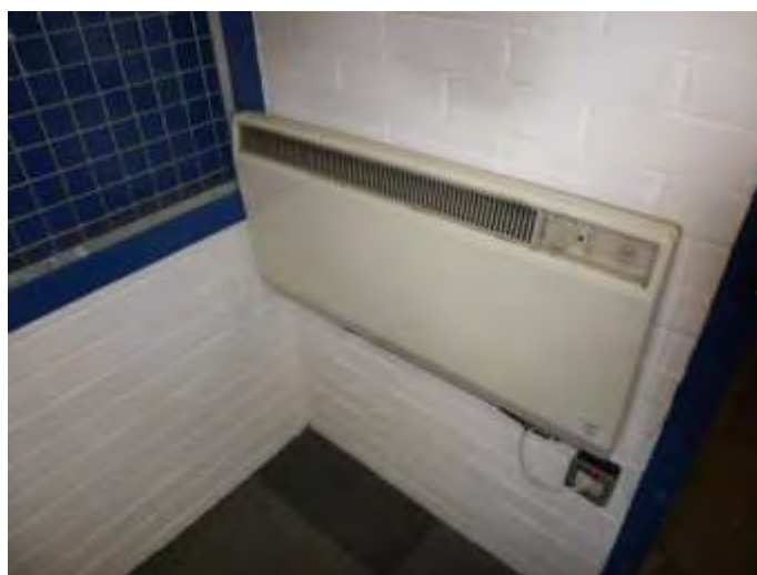
Modern Heater in Security Office
