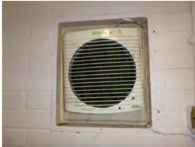
Plastic Extractor Fan to Staff WC
