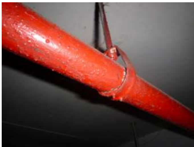
Metal Sprinkler Pipes on Metal Hangers
