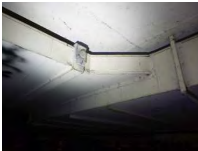
Metal Ducting to Ceilings
