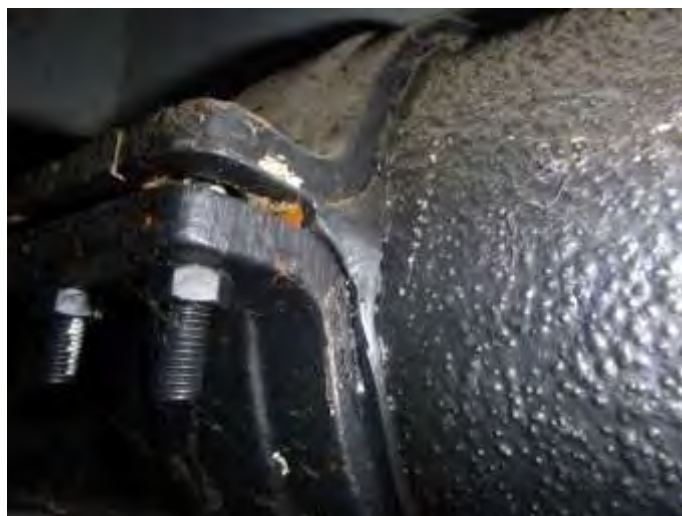
Rubber Seals to Cast Pipes within Car Park
