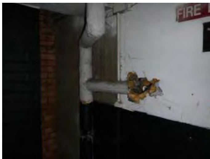
Rockwool Pipe Insulation near Roller Shutter Door on Upper Level
