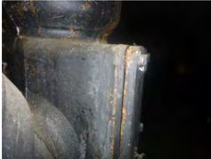
Rubber Seals to Pipe Access Panels
