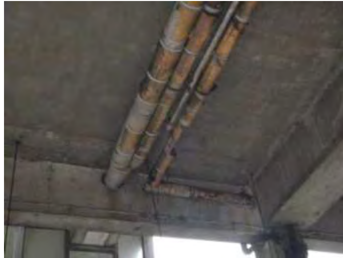
Rockwool Pipe Insulation at High Level above Vehicle Entrance
