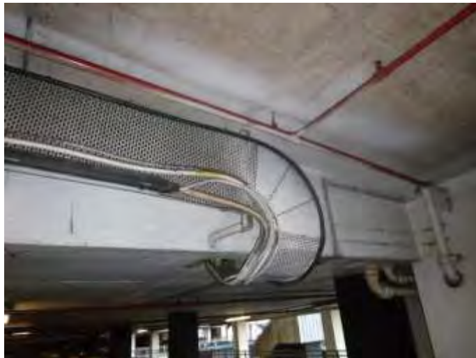
Steel Electrical Cable Tray
