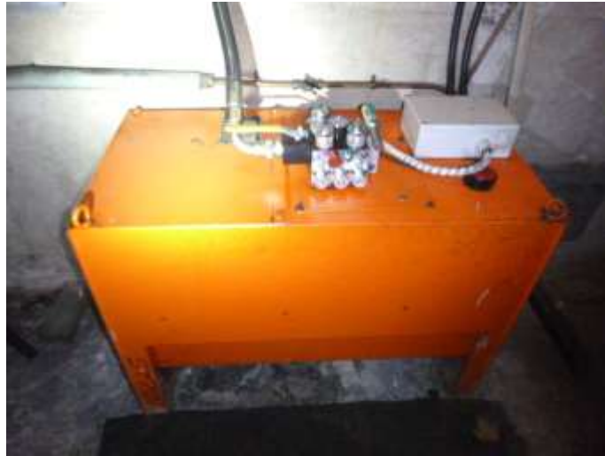
Hydraulic Lift Motor to Hotel Laundry Lift
