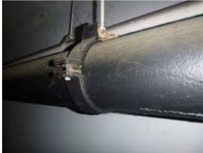
Metal Hangers to Cast Pipes
