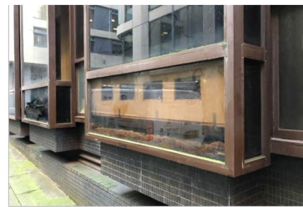
Photograph No. 24 – Ground floor exposed spandrel glass panel with black coating diminished – (Ground floor – North elevation – Marsden Block)
