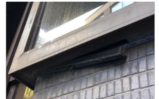
Photograph No. 29 – Impregnated foam found loose between façade and glazing system (Level 1 – West elevation – Marsden Block)
