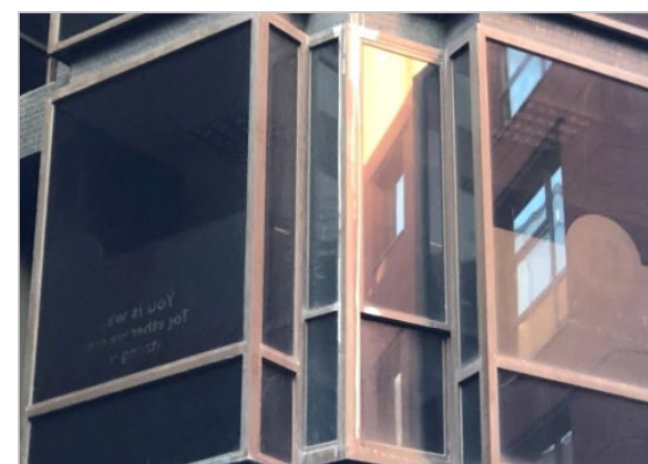
Photograph No. 19 – Excess water staining observed to corner bay (Level 3 – West elevation – Marsden Block)
