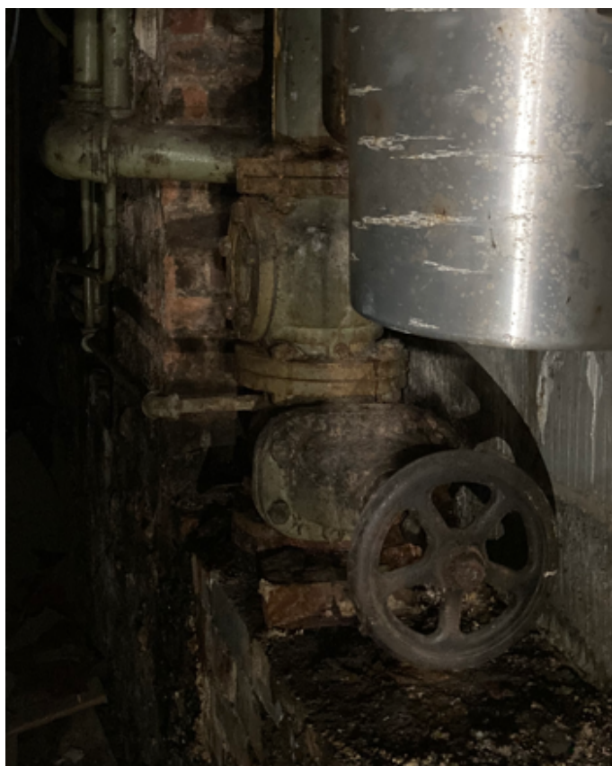
Photo 6: Extensively corroded alarm valve
