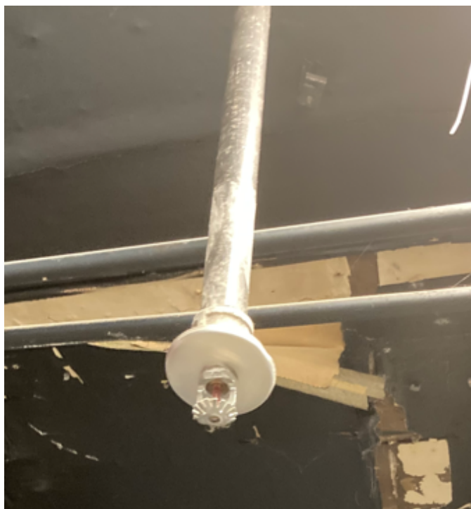
Photo 5: Modern sprinkler head and pipework
