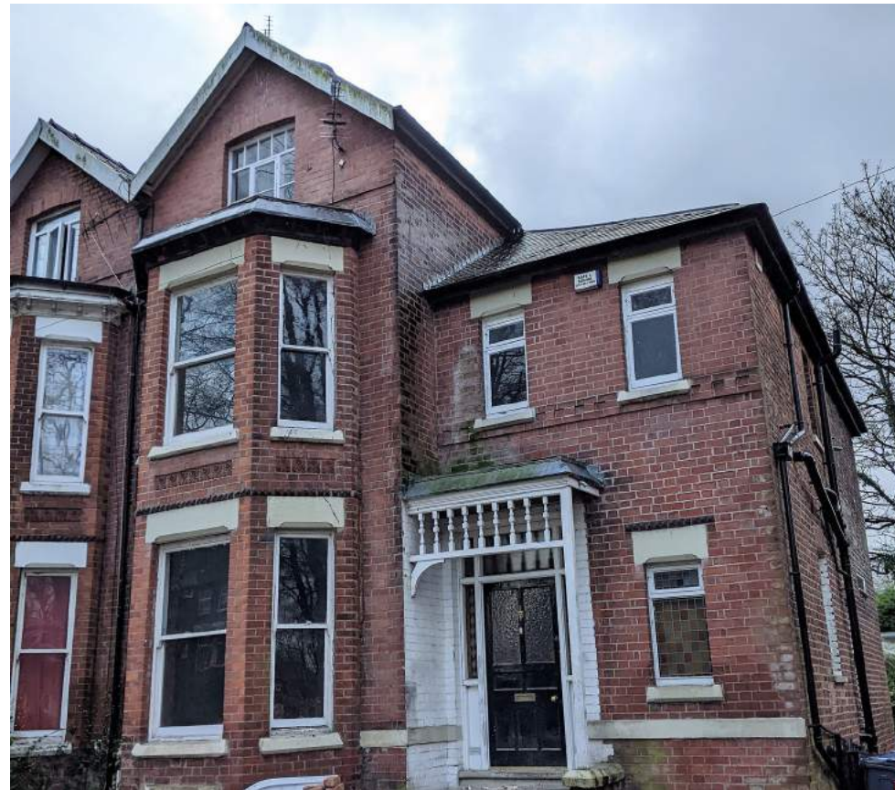
Front elevation of property, where the bay window has suffered from severe subsidence
