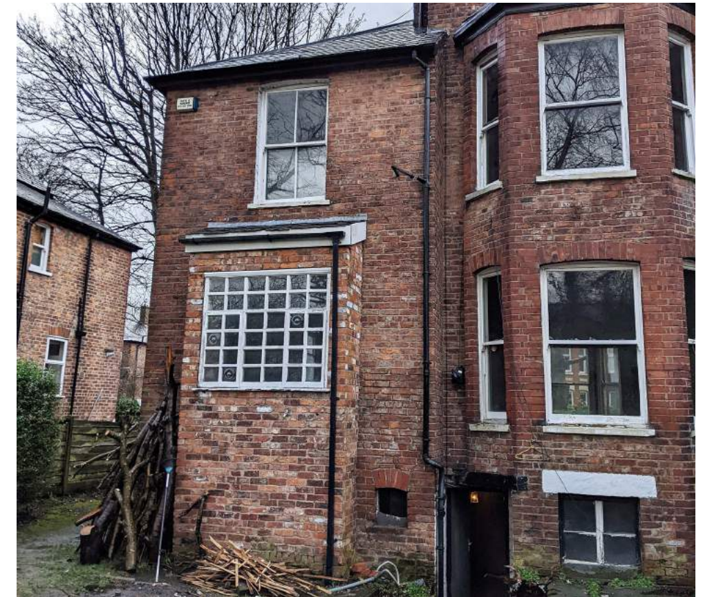
Rear elevation showing poor quality extension with incongruous 'Georgian' style window
