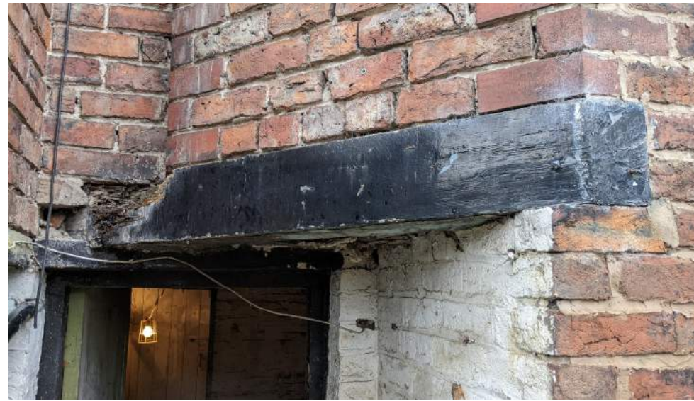
Rotten timber lintel to rear bay window at basement entrance
