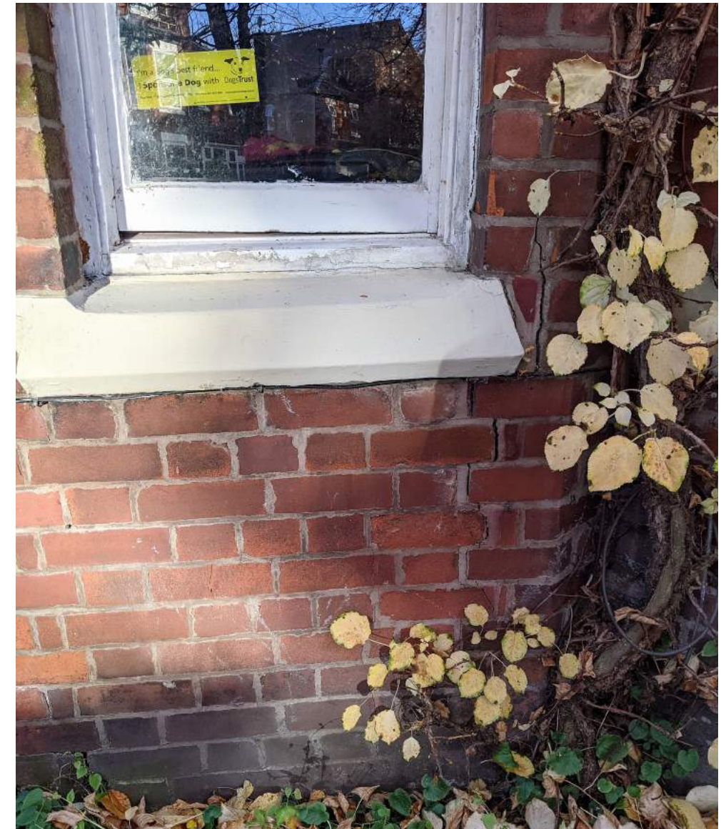
Bay window, showing distorted window opening and cracked brickwork due to severe subsidence
