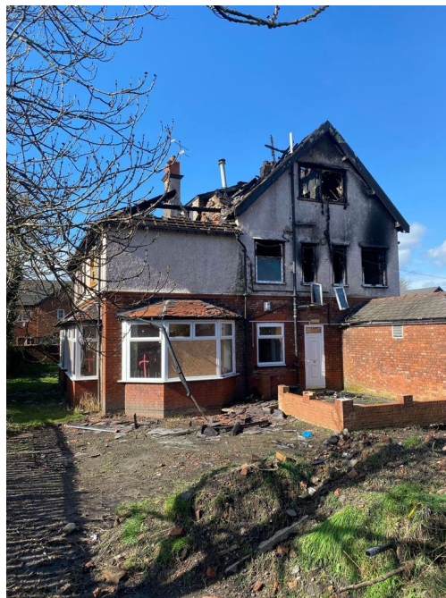
Photograph 2 – Building 1a following arson and fire damage.
