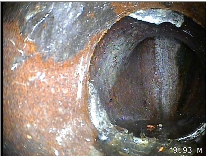
Line of drain/sewer deviates up
