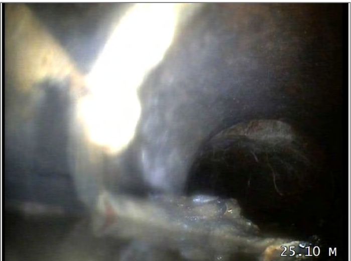
Settled deposits coarse 15% cross-sectional area loss
