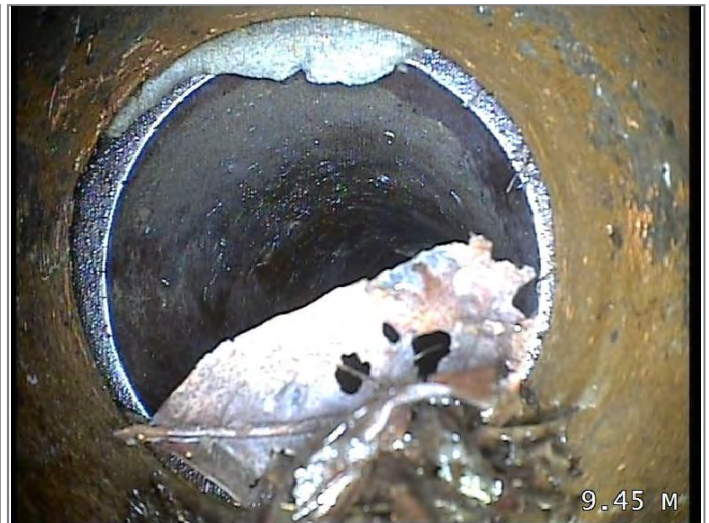
Joint displaced medium - Remark: SEAL VISABLE
