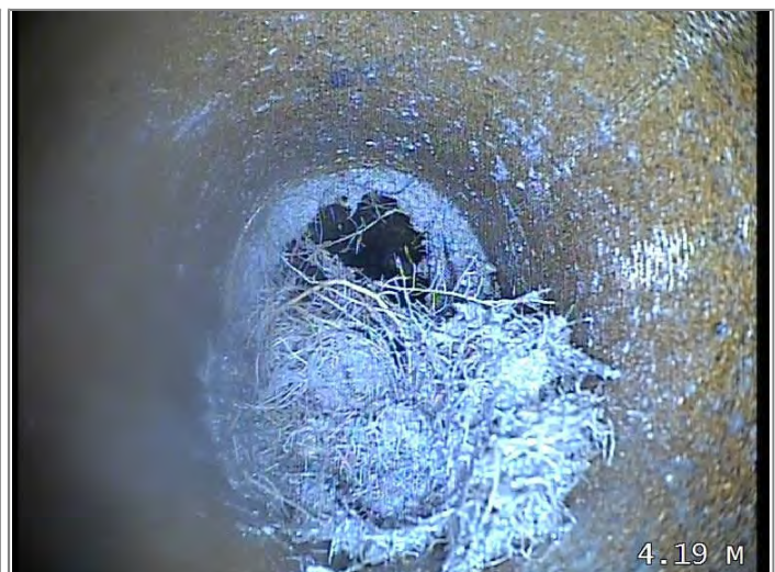
Roots mass 50% cross-sectional area loss
