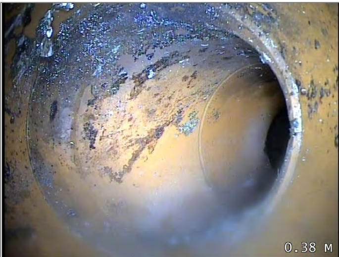
Line of drain/ sewer deviates right
