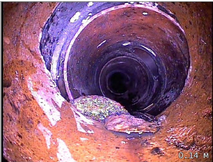
Hole in drain/sewer from 8 to 12 o'clock - Remark: PIPE BROKEN - REPAIR NEEDED
