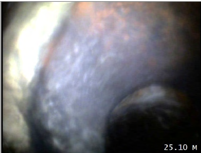
Joint displaced large
