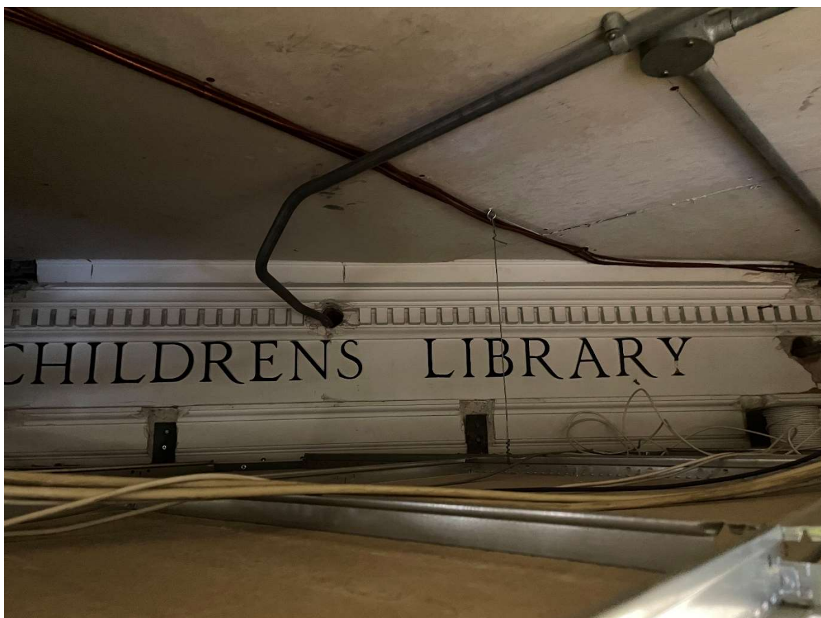
Some of this has been hacked about to insert beams for the floor, route services and fix the ceiling trim.
