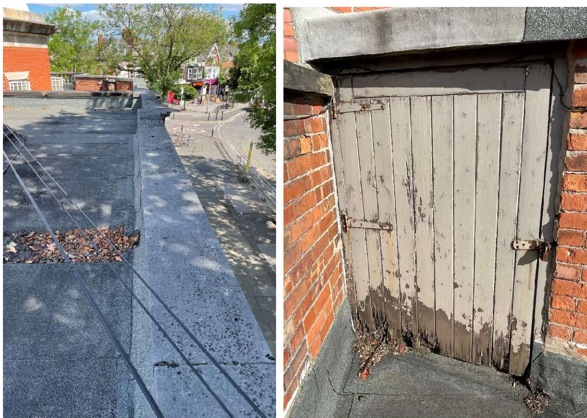
Looking north along the east parapet wall, and the decayed Tank Room door to be replaced.
