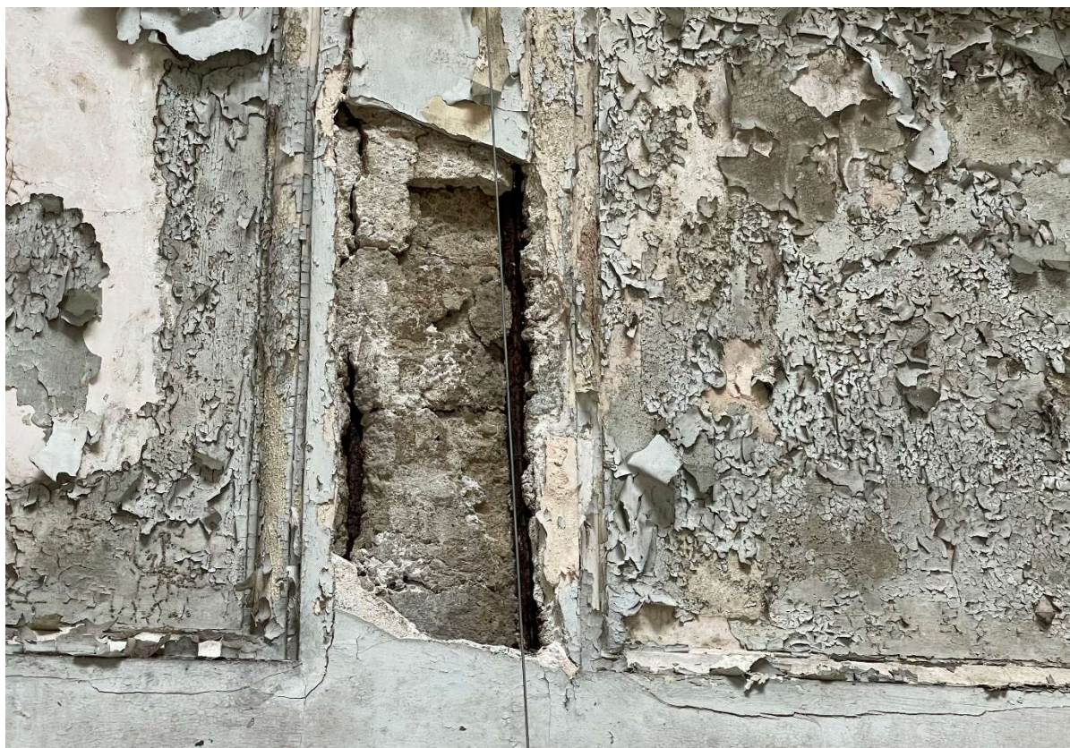
Specialist repair required to corroded reinforcement in the centre of the south facet.
