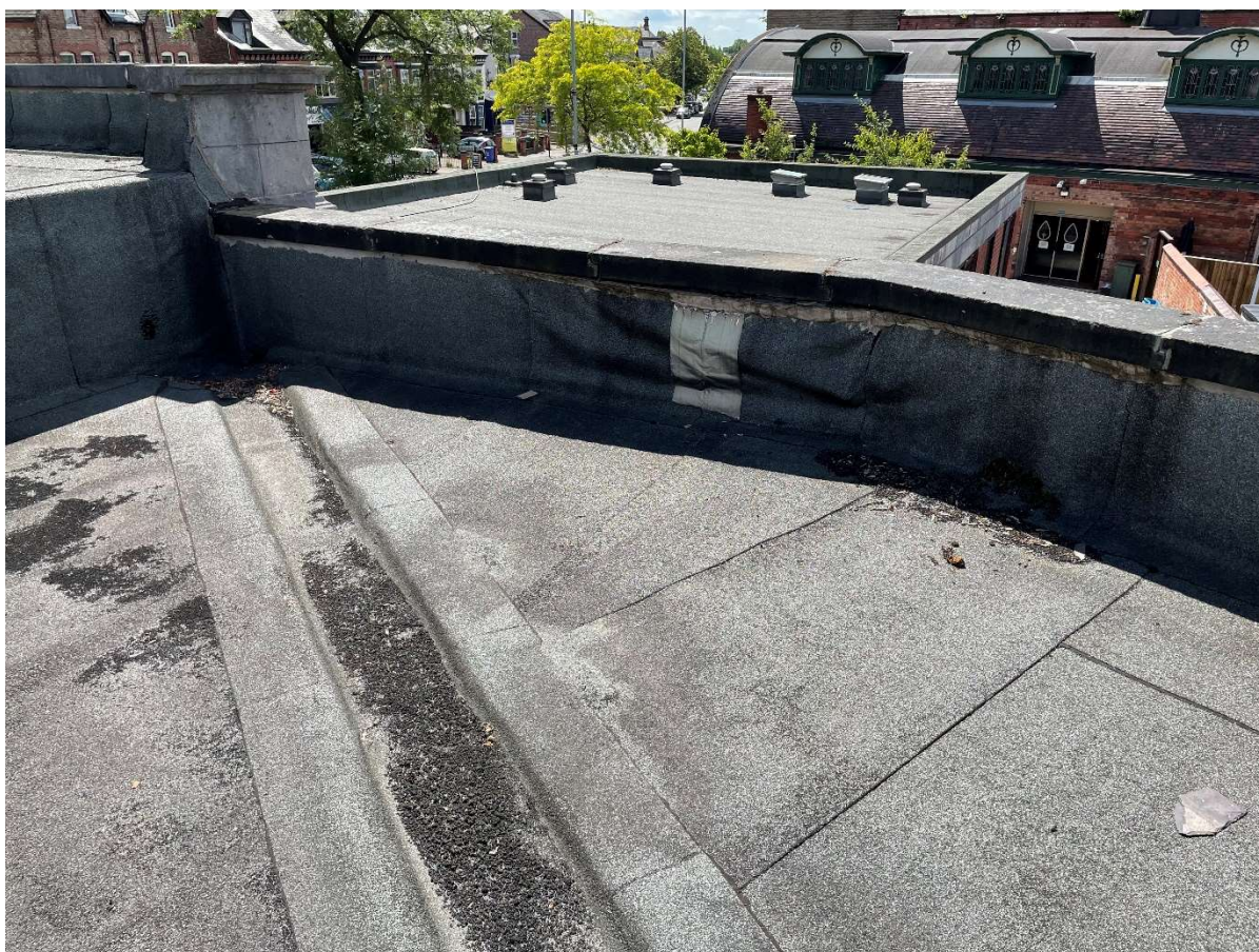
Area of sagging felt to be renewed, rear of south-west parapet wall, with the extension roof behind.
