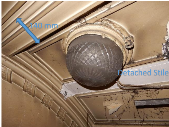
Photo 5: Showing the framed square ribs / stiles which run along the length of the ceiling, one of which has become detached; also showing the small planted on square section, creating a frame to the inner panel; and the cut glass light fitting.
