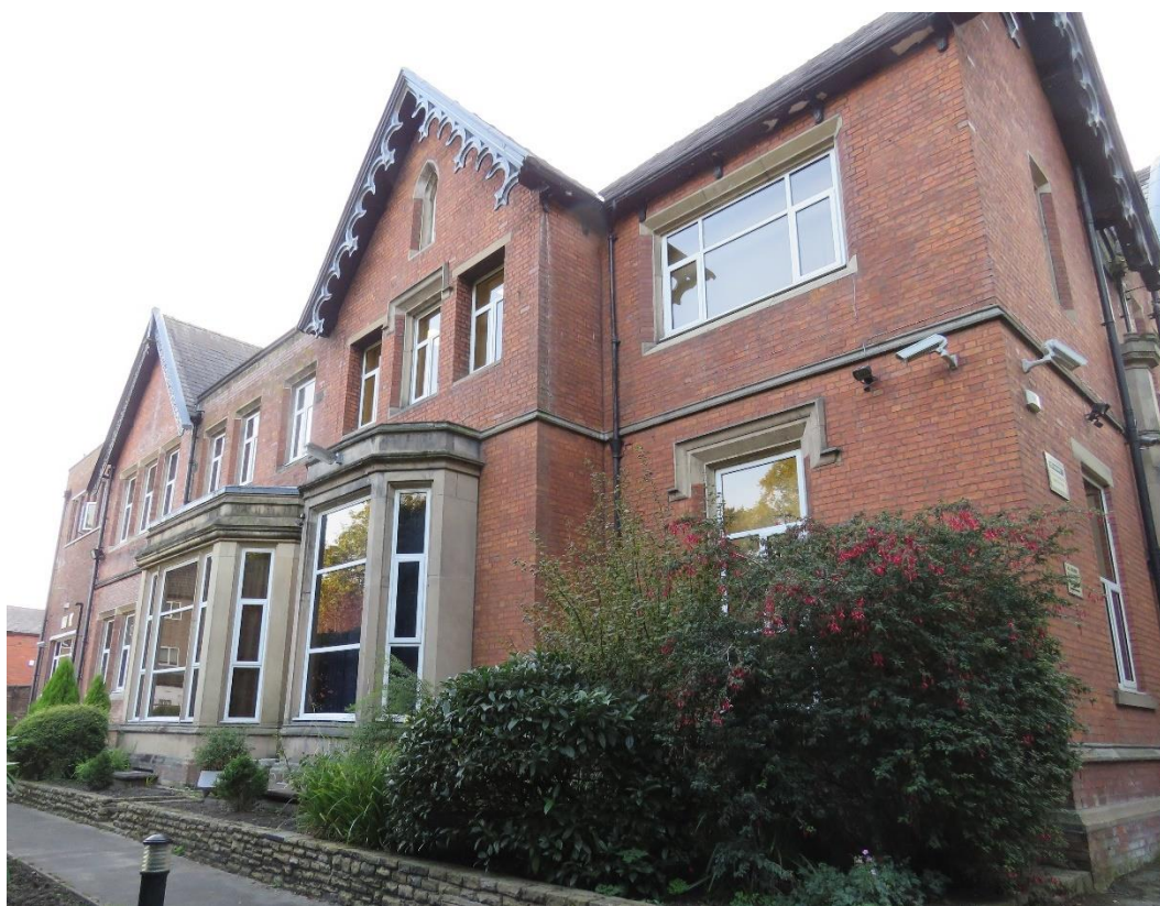
Figure 42 – The east elevation as seen in 2020 showing the subsequent removal of the original Gothic stone mullions to both ground floor bay windows.
