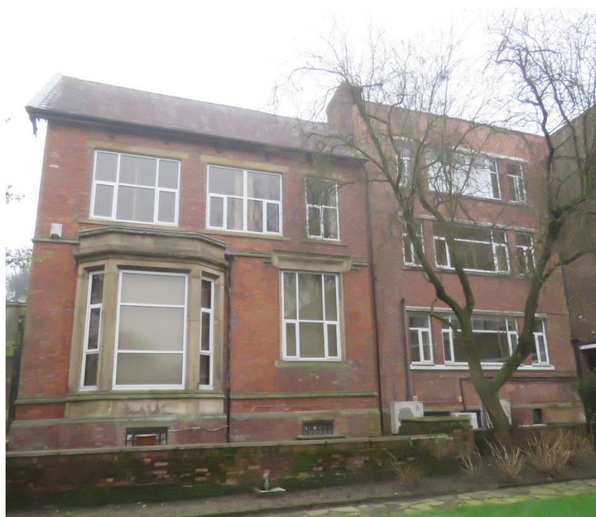
Figure 39 – The same view as seen in 2020, showing the subsequent removal of the stone mullions from both ground floor windows and poor quality uPVC windows that detracts from the architectural appearance of the house.
