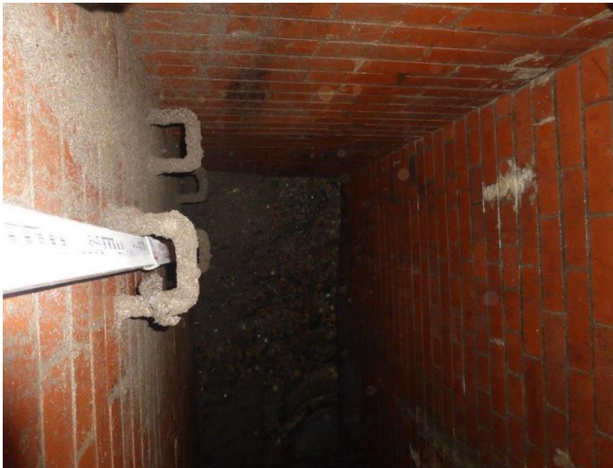
Figure 3-3-Abandoned chamber found during GI
