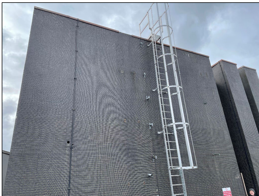
Photograph A2.2: Central column, housing utilities, located on the central roof.
