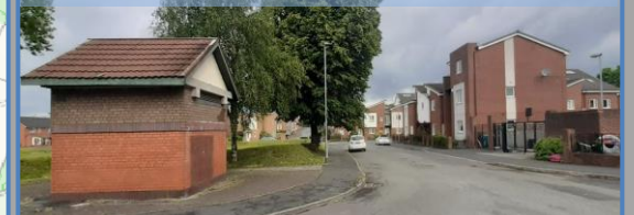
A sub-station housed in a brick shed at the eastern edge of the site next to Stracey Street
