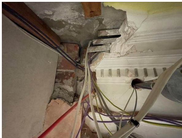
Lost and damaged plaster details to be reinstated.
