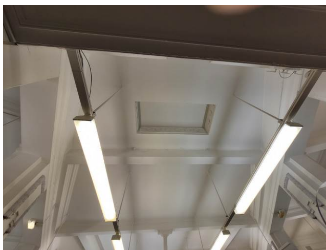
Existing lighting suspended on trunking.
