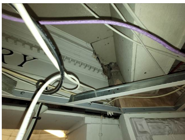
Gallery support detail lost when steel beams inserted.
