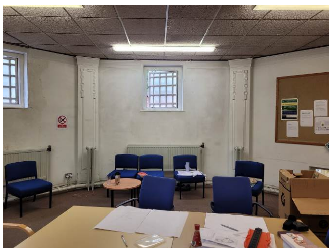
Corner column radiators in the staff room.
