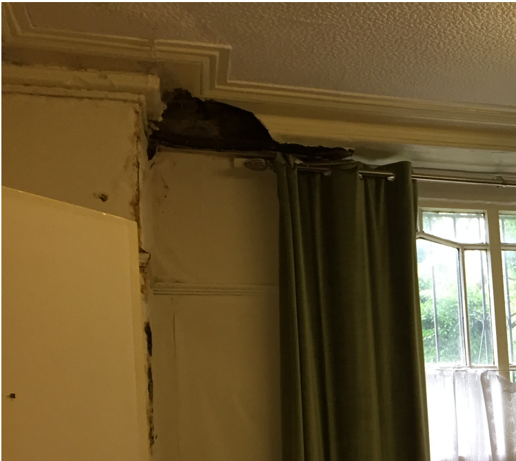
Partial collapse of coving to proposed dining room
