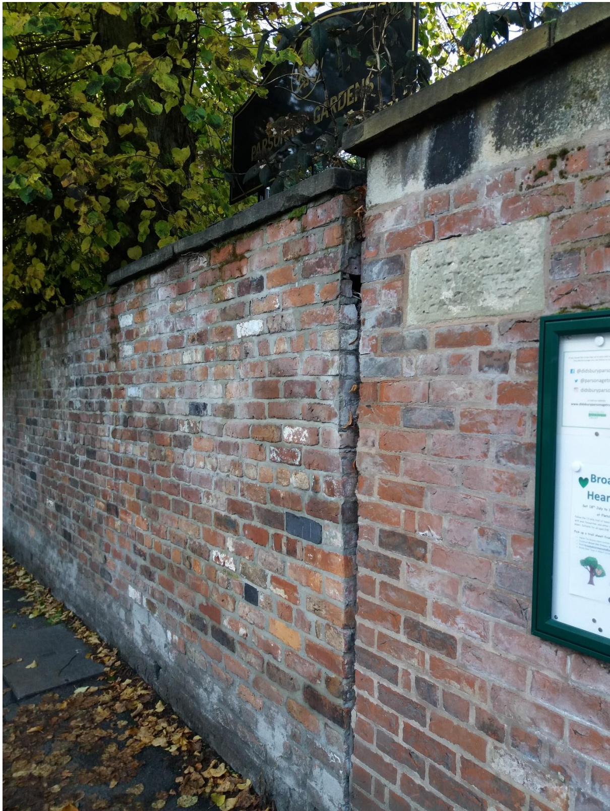
Photo 2: Leaning boundary wall close to stone arch entrance on Stenner Lane.
