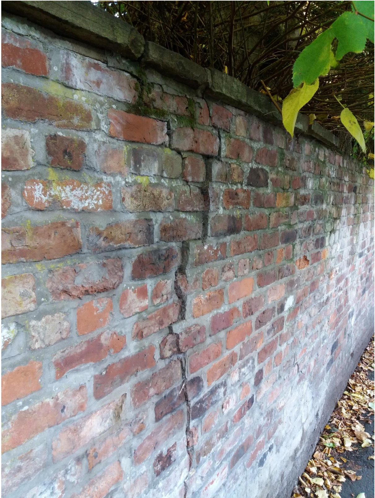
Photo 4: Photograph of cracking to boundary wall caused by tree growth and movement. Location of emergency works to reduce the wall height by 9 courses of brickwork, undertaken in June 2021. See Photo 5 for final finish.
