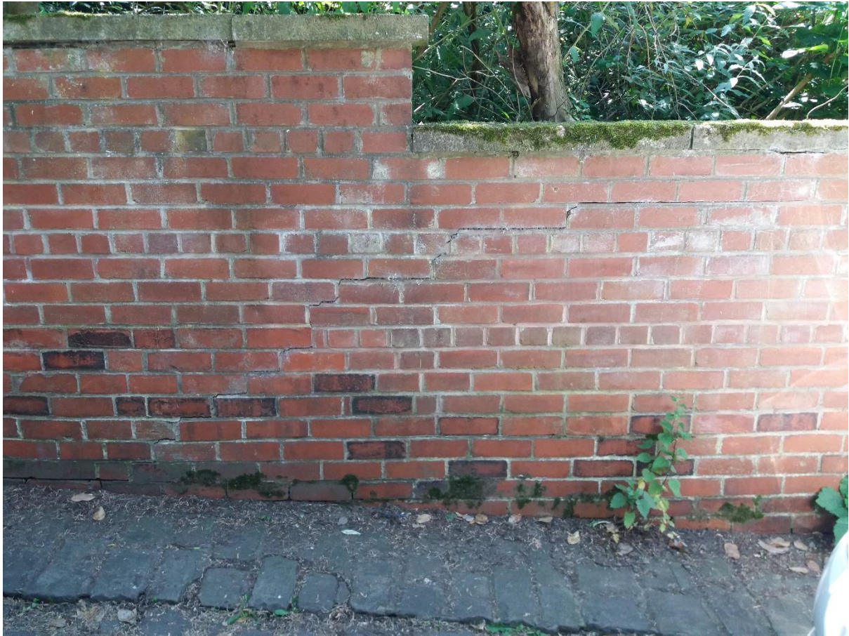
Photo No.12: Stepped cracking to boundary wall on western side of Stenner Lane adjacent Fletcher Moss Park.
