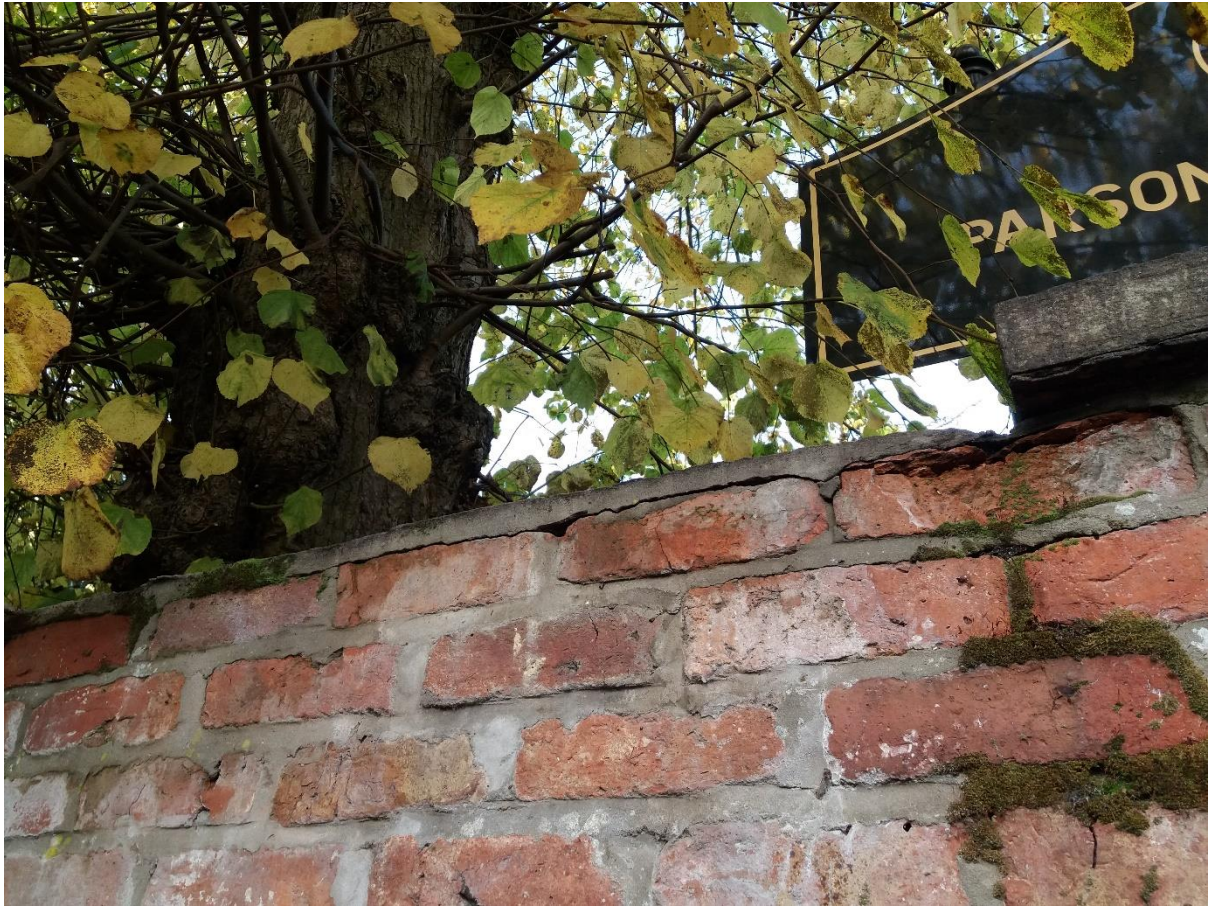
Photo 8: Missing Coping stones; the sandstone coping stones are missing to the majority of this section of wall on Stenner Lane
