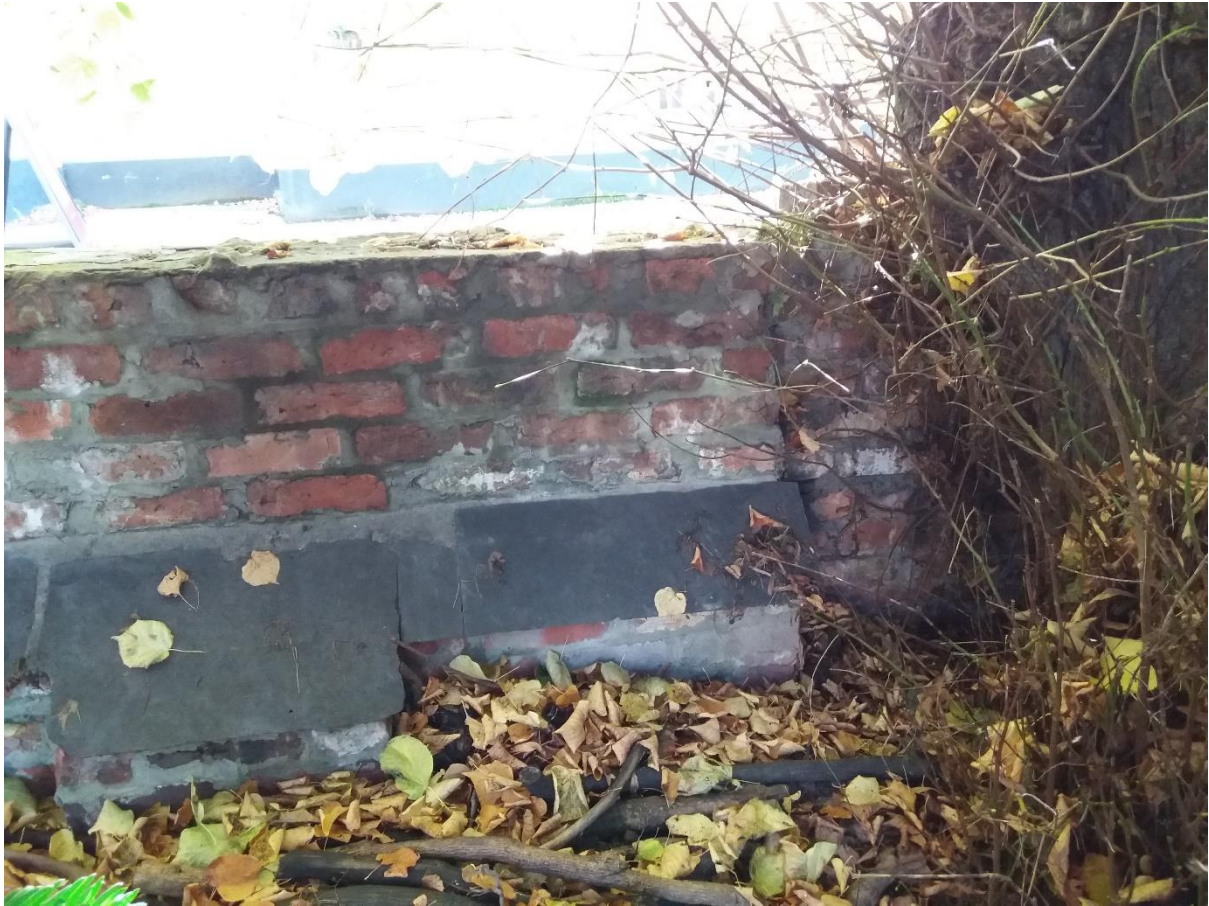
Photo No.9: See changes in wall thickness from top of boundary wall down to increased thickness at ground level.
