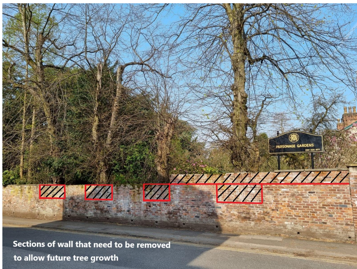
Photo No.10: Highlighted sections of wall that need to be permanently removed to allow the trees space for future growth.
