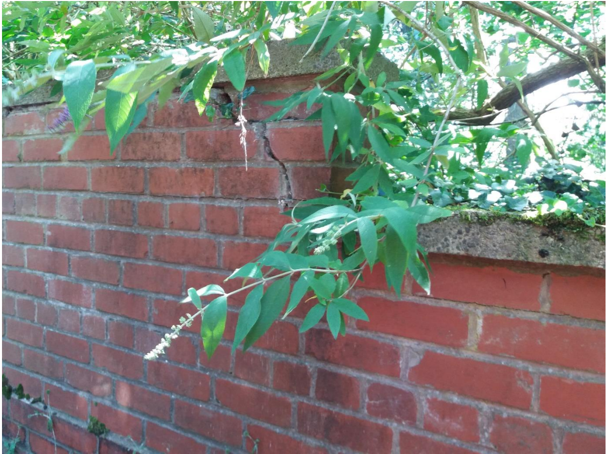
Photo No.11: Damage to section of boundary wall to Fletcher Moss Park to Western side of Stenner Lane.
