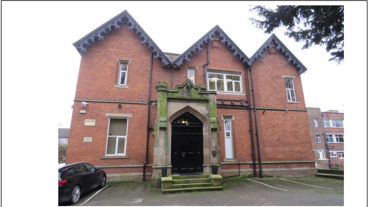
Figure A – The original entrance to the principal north elevation. Note the uPVC windows which detract from the appearance of the former house.
