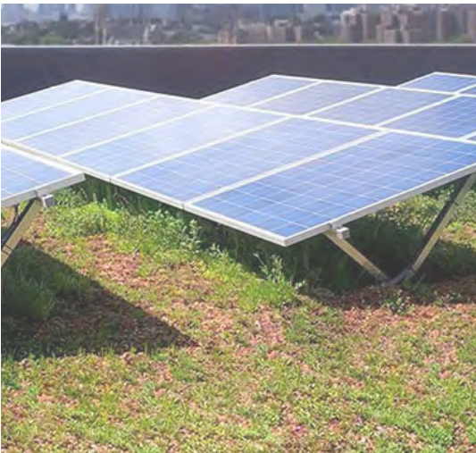
Renewables: Photovoltaic Panels
