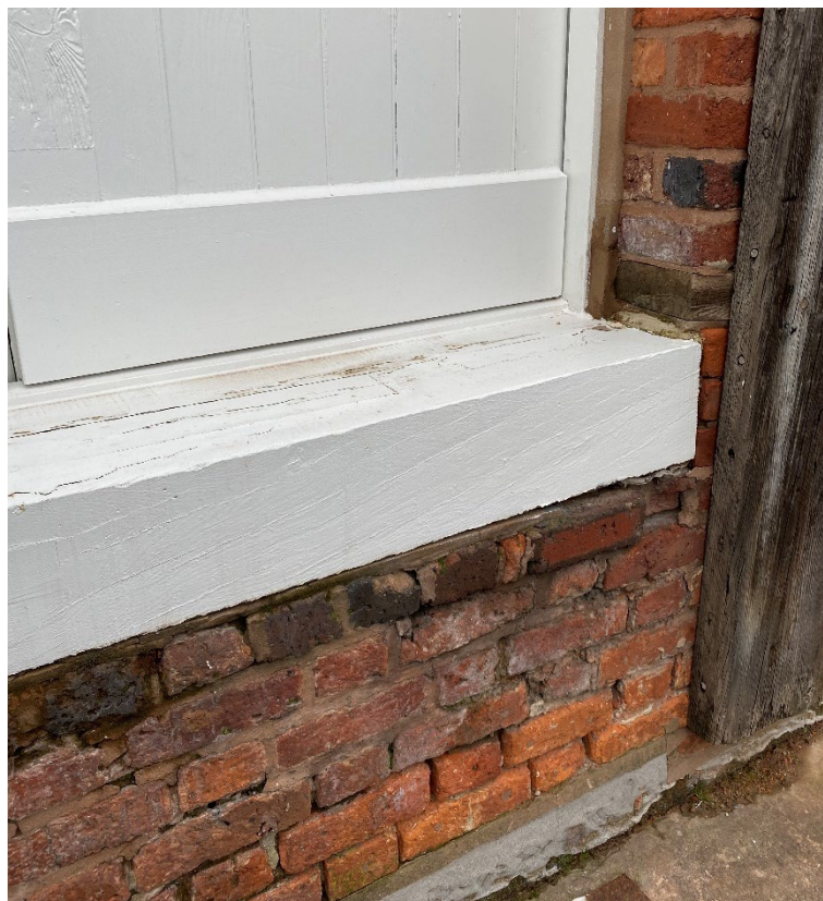
Figure 10: timber lintel on south façade showing past pieced in repair to upper surface, and damage and discolouration to historic brickwork beneath.
